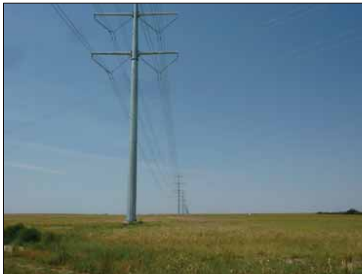
Photo 5.26-1. A transmission line present in the Action Area.
