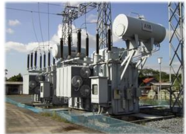
Generator Step-Up Transformer
