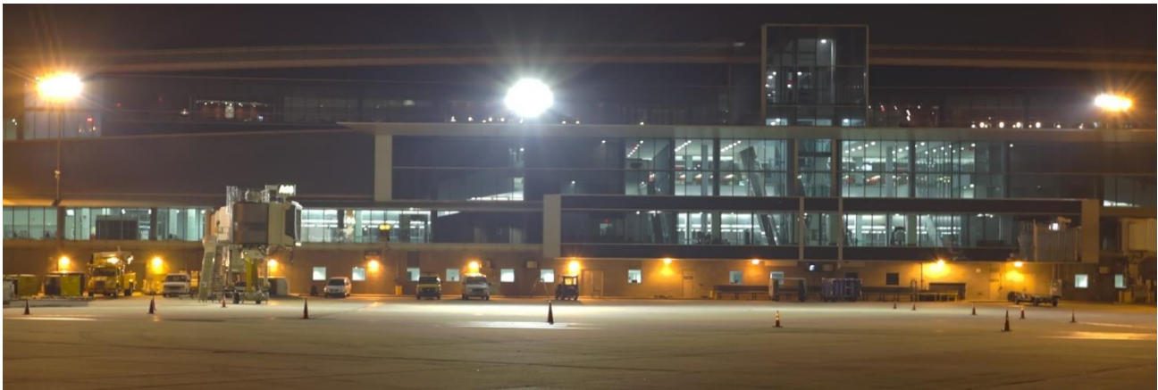
Figure 6. Photo of the second trial installation of LED luminaires on pole 16. The difference in CCT (2200 K for the HPS vs. 4000 K for the LED) is apparent, particularly on poles 15 and 17. All LED luminaires were mounted at a 70° tilt.
