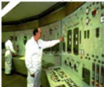
Plant Status Display
