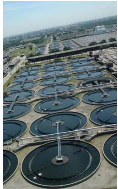
Stickney Water Reclamation Plant, Chicago
