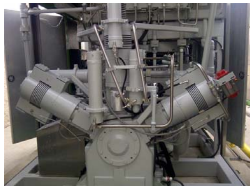
View of Compressor inside enclosure
