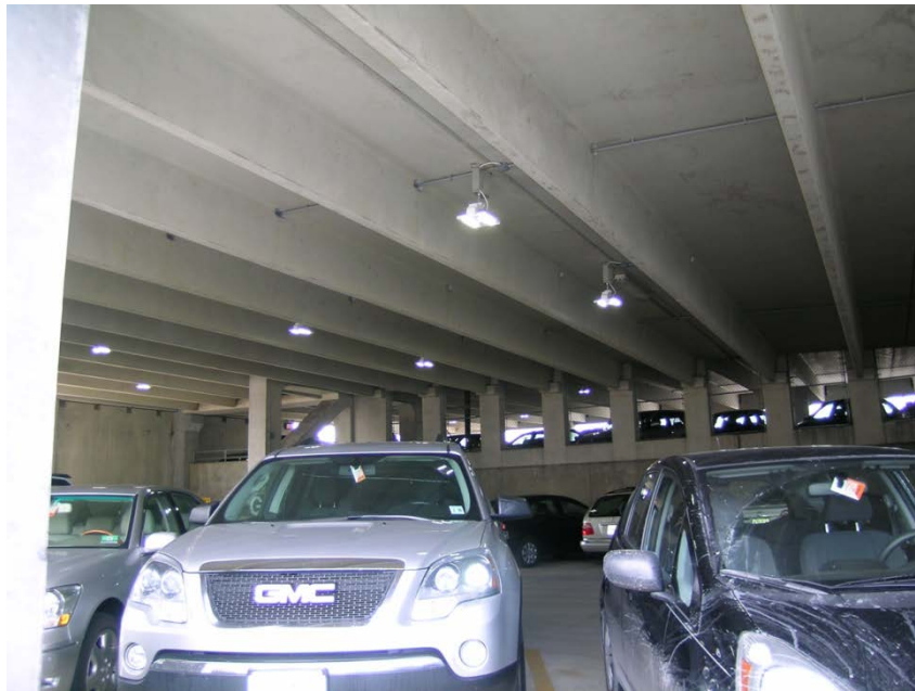
Figure 13: LED luminaires installed in the West Garage.
