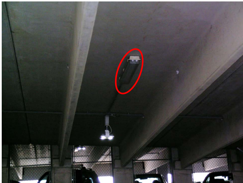
Figure 14: An existing fluorescent luminaire (shown in OFF condition), still used for emergency lighting.
