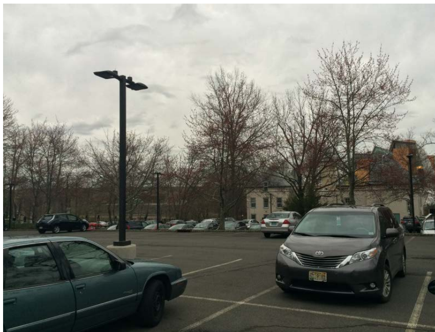
Figure 18: Location and photo of parking lots converted to LED in phase two.
