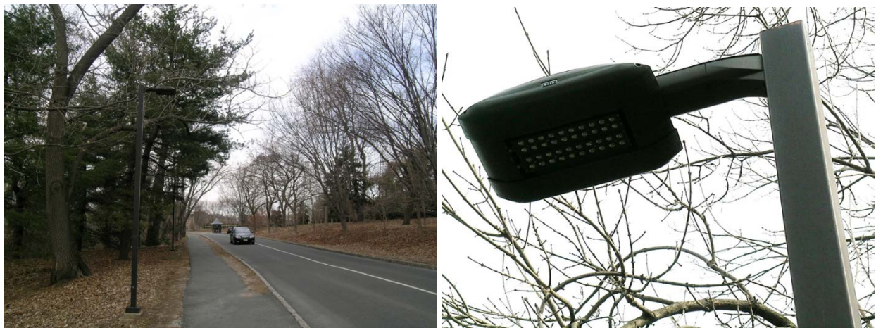
Figure 6: New LED luminaires along Elm Drive, looking north towards the Guard station at the South entrance (left) and a close-up view (right).
