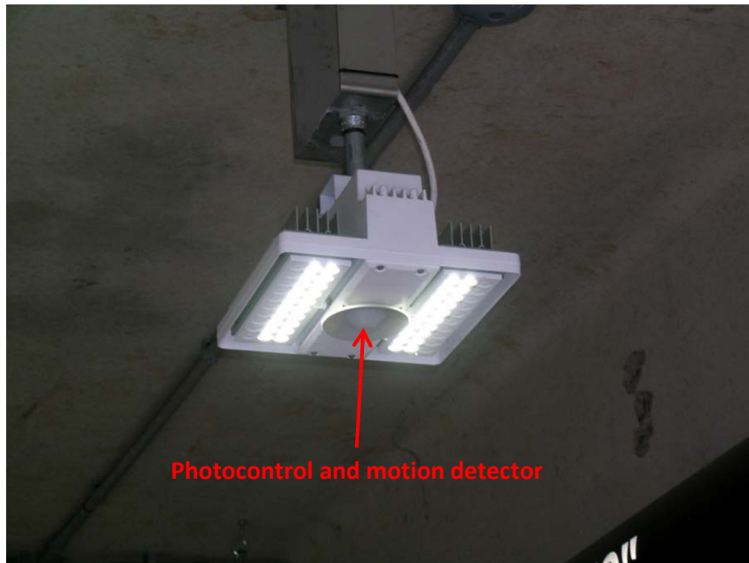
Figure 15: Close-up view of an LED luminaire, with the photocontrol and motion detector in the center of the luminaire.
