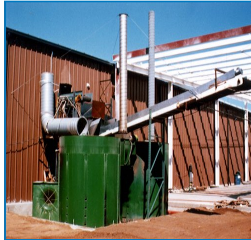
Biomass Heat Exchanger NREL/PIX 03447
