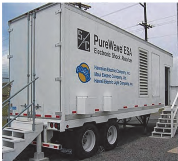
Figure 2-67. Ultra Capacitor Installation
