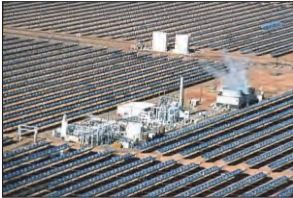
Figure 2-38. Parabolic Trough Solar Farm with High-Temperature Solar Collectors and Support Facilities, Cooling Towers, White Water Tanks, and Generation Equipment (Source: DOE-EERE 2013b)
