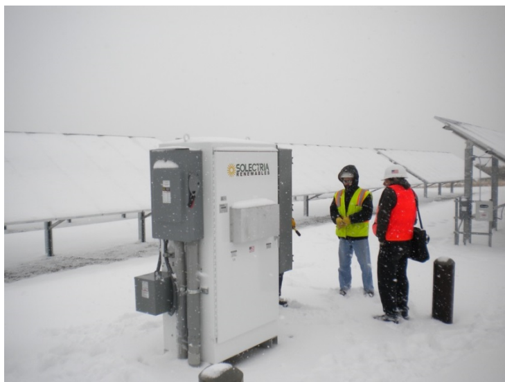
Inspection of a PV system at Mesa Verde National Park. Photo by Andy Walker, NREL
