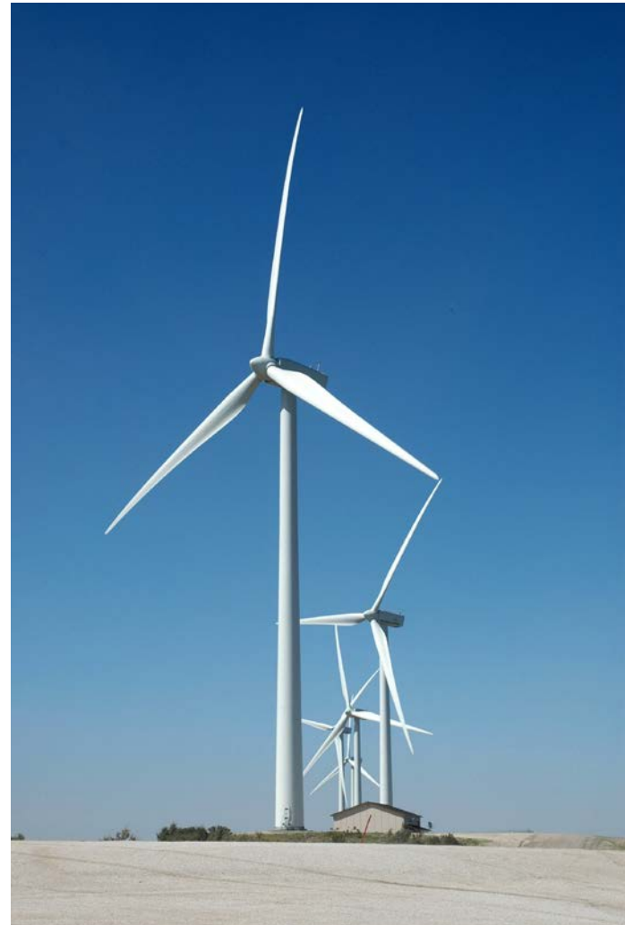
Wind power project at Campo Reservation about 60 miles east of Sand Diego, California. Photo by Robert Gough, NREL 6312056.
