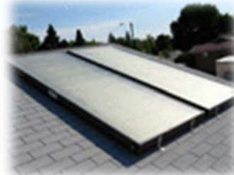
Solar Water Heating
