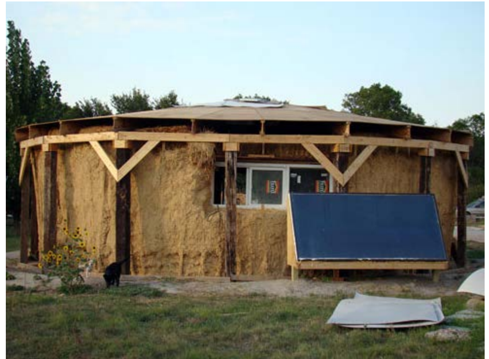
Straw bale housing with solar heating at the Red Cloud Renewable Energy Center in Pine Ridge, SD.
