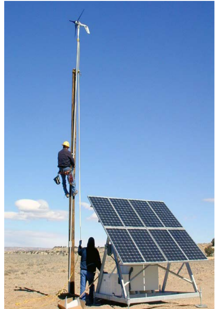
Members of the Navajo Tribal Utility Authority install a wind turbine. Photo by Larry Ahasteen.
