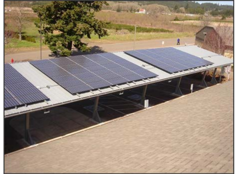
PV panels installed on Grand Ronde Tribal Housing Authority carport. 42 kW: Combination of tribal funds and state incentives Photo from GRTHA, NREL 31797
