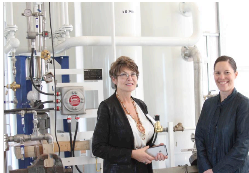
Blue Lake Rancheria Vice Chairperson Aria Ramsey and Energy Director Jana Ganion at the Tribe's biomass-to-fuel cell power plan. Photo from Jana Ganion, NREL 32766
