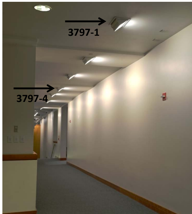
Figure 14. Hallway 3797 Photograph: LED Initial. The photograph shows the seven large wall washers in the foreground, with additional large wall washers over the stairs, illuminating the background. Wall washer 3797-1 was installed in August 2014, and the remaining wall washers in 3797 were installed in March 2015. Illuminance measurements were recorded for the wall and floor areas near 3797-4.
