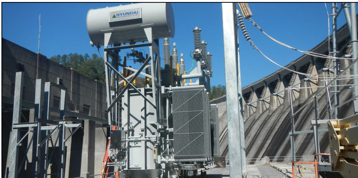
One of the two power transformers replaced at the Allatoona Project utilizing customer funding. The $17.8 million effort includes a complete reconfiguration of the switchyard, replacement of the 115kV circuit breakers, associated bus work, superstructure and added new 13.8kV generator breakers.
