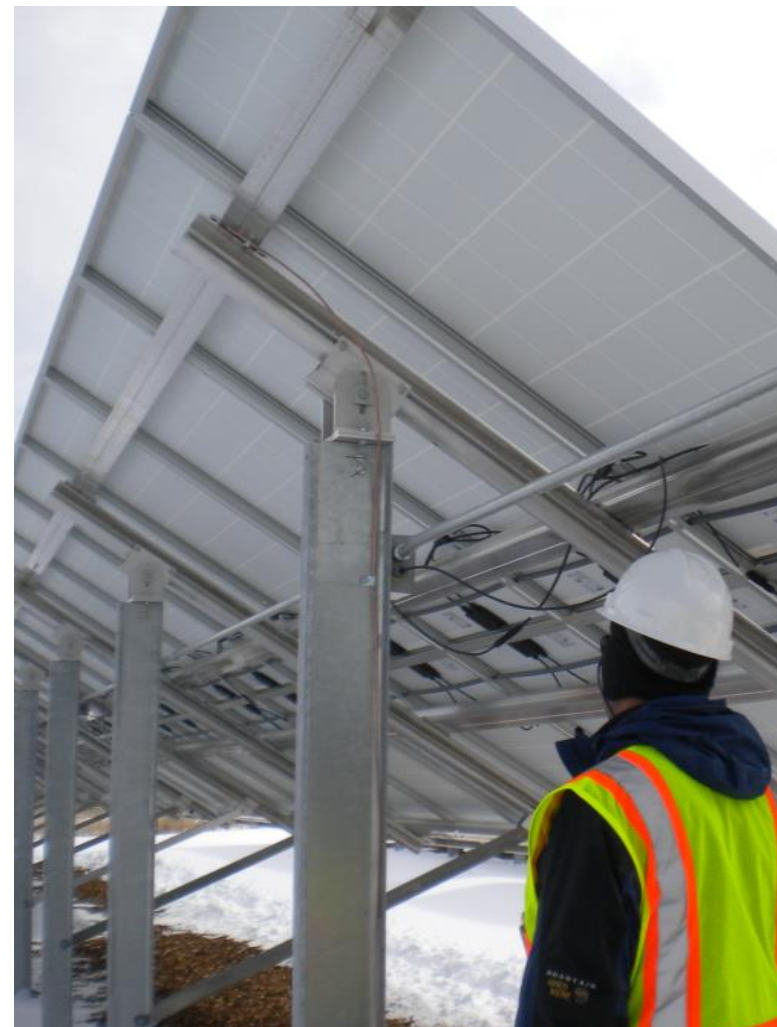
Inspection of a 67-kW PV system at Mesa Verde National Park. Photo by Andy Walker, NREL
