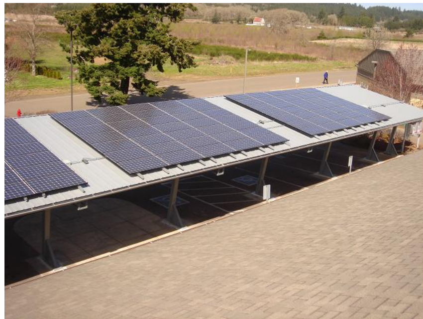
PV panels installed on Grand Ronde Tribal Housing Authority carport. Photo from Grand Ronde Tribal Housing Authority
