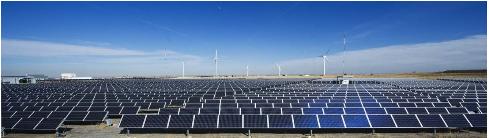
1 megawatt of solar PV at NREL's National Wind Technology Site. NREL 19794
