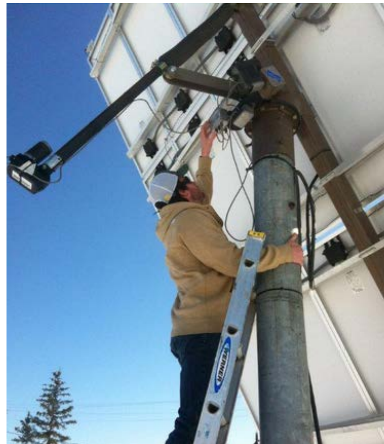
Photo by Brian Hirsch, NREL 20893
