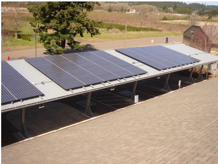
PV Panels on Grand Ronde Tribal Housing Authority carport. Photo by GRTHA, NREL 11659046
