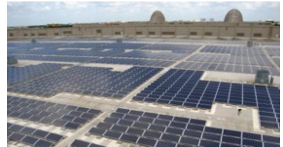
Orange County Convention Center, NREL 18077
