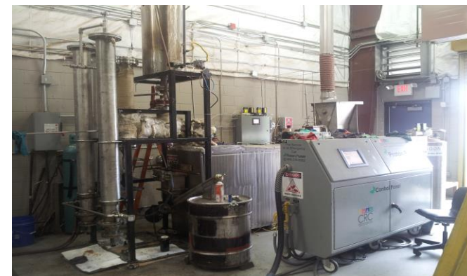
Pilot auger pyrolysis reactor at UTK Center for Renewable Carbon
