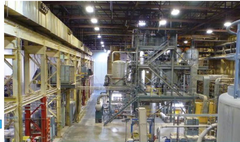
Figure 1: Ensyn has recently enhanced its Ontario facility, converting it to a dedicated fuel facility with a capacity of three million gallons/year.
