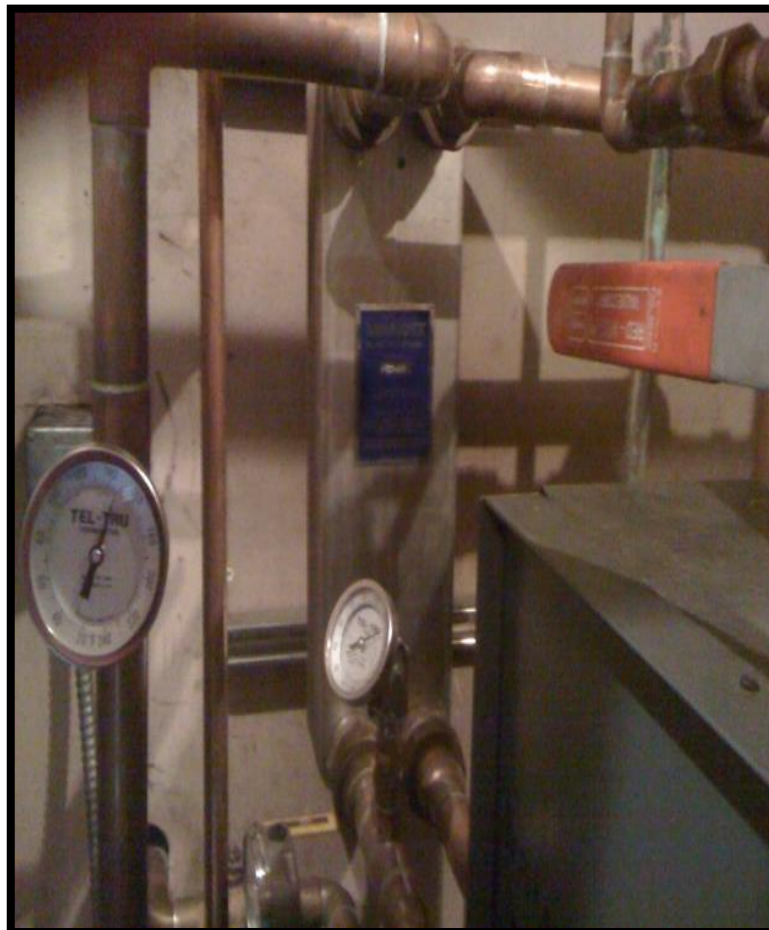
Boiler Room Heat Exchanger
