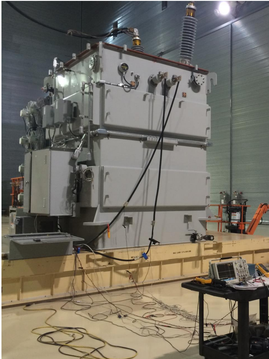
Prototype (1-Phase) 7.5 MVA CVSR Under Test at SPX
