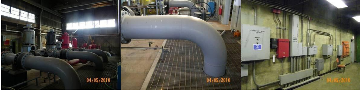
Fig. 7. X-626-1 Pump House pump room, header trench, and control panels.
