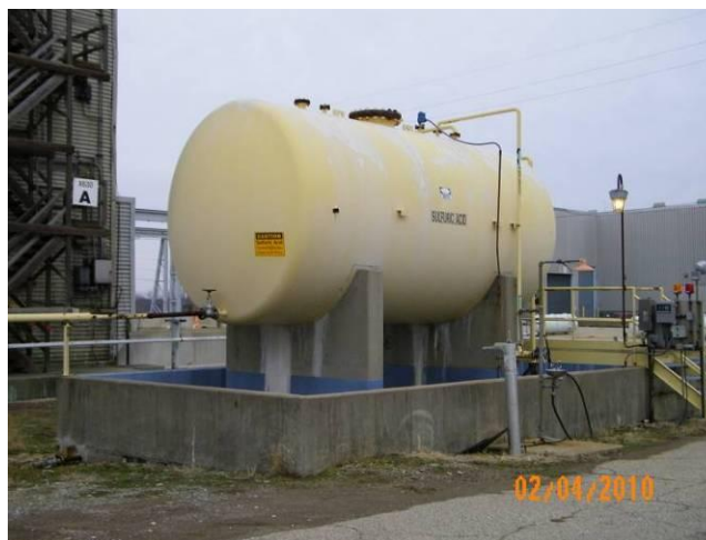
Fig. 16. X-630-3 Acid Handling Station
