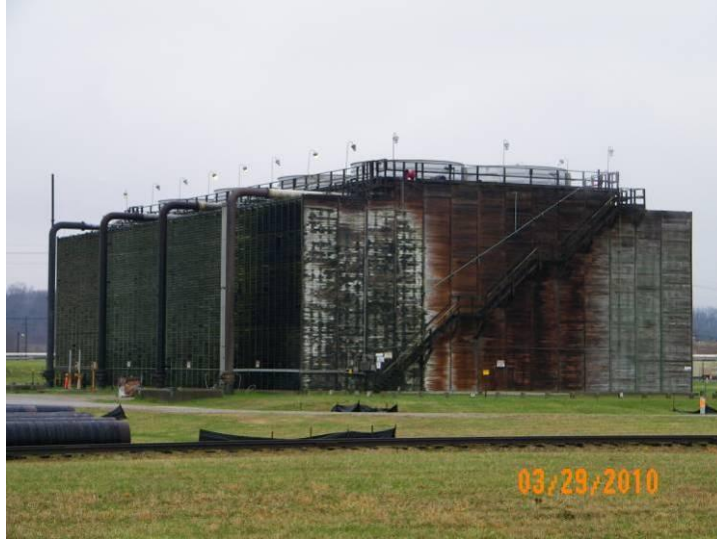
Fig. 8. X-626-2 Cooling Tower.
