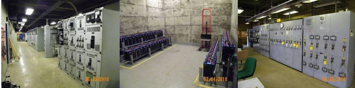
Fig.14. X-630-1 switchgear room, battery room, and control area.
