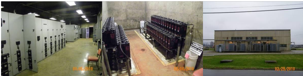
Fig. 6. X-626-1 Pump House switchgear room, battery room, and transformer platform.
