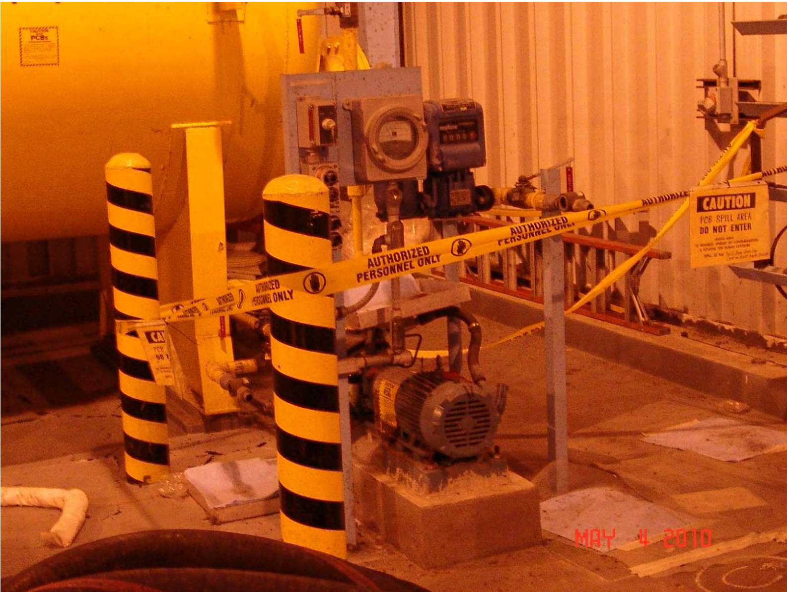
Figure A.5. Building X-334 - area roped off as PCB spill area.
