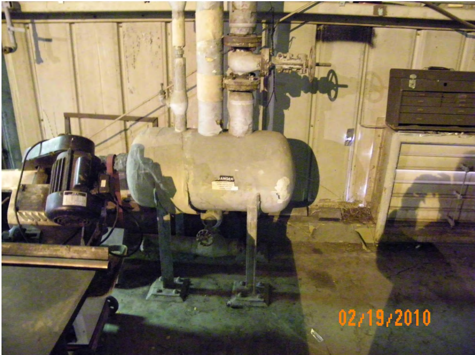
Figure A.8. Building X-344B - equipment/pipe with asbestos insulation.
