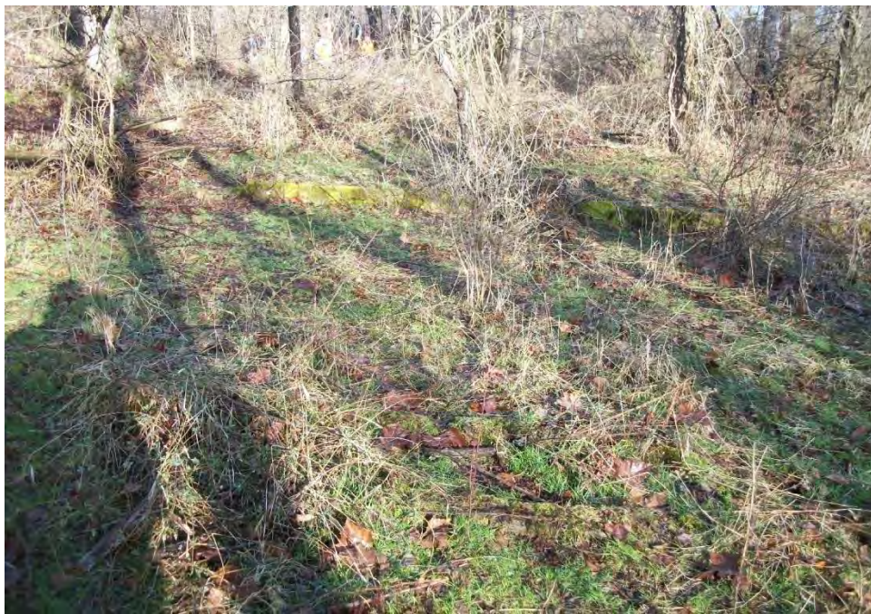
Plate 24. Overview of HMBL 4 showing the edge of the concrete milk barn foundation remnant; facing north-northwest.
