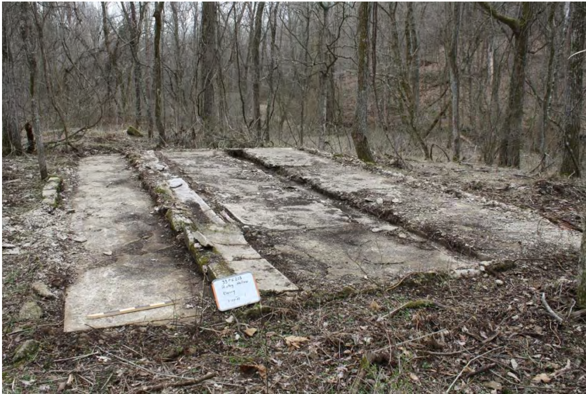
Figure 70. Photograph of a poured concrete milking platform at Ruby Hollow Farmstead (33Pk203).
