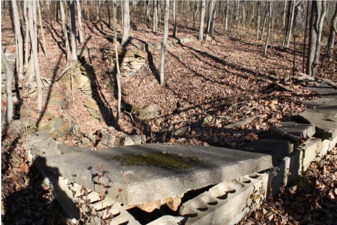
Figure 67. Photograph of a rough fieldstone masonry cellar foundation (background) with cinder block and poured concrete (foreground) at Brodess Farmstead (33Pk311).
