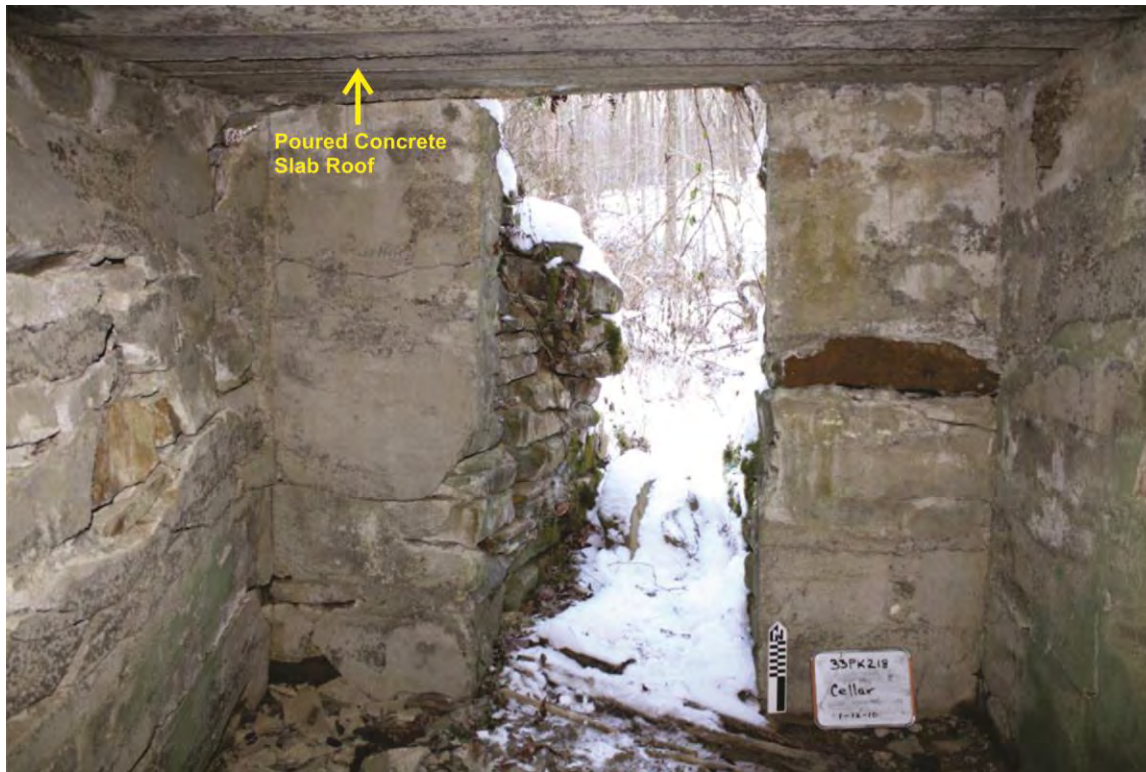
Figure 72. Photograph of a poured concrete slab roof (stone masonry walls have mortar skim coat) on external root cellar at Cornett Farmstead (33Pk218).
