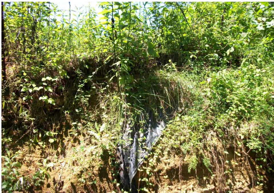
Plate 22. Geotextile and fill along the bank of the small creek east of HMBL 41; facing north-northwest.
