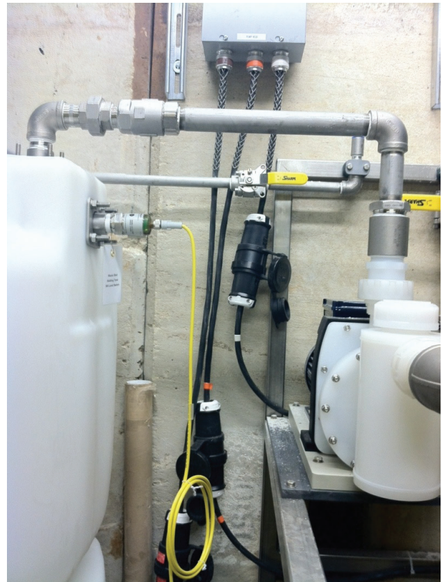
Exhibit 4-7: MI-65 Service Building Exchange Skid Electrical Quick Connects/Disconnects
