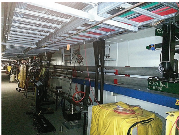
Exhibit 4-6: Cable Tag Location for Cable Destination
