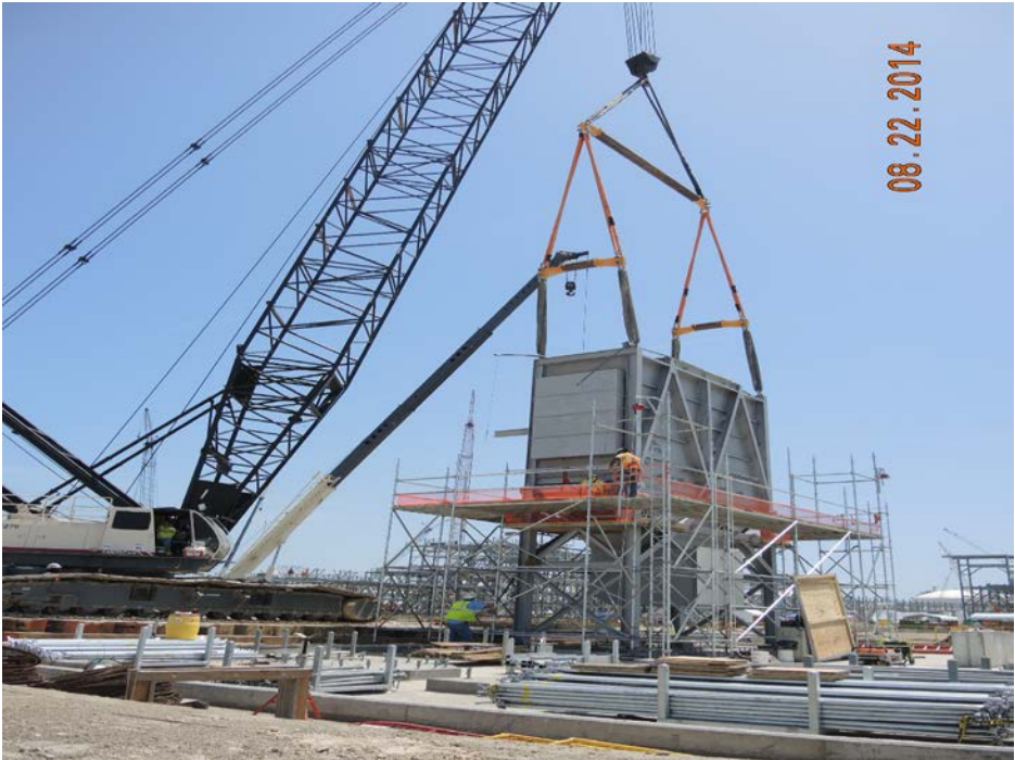
OSBL2 Setting Thermal Oxidizer Heat Recovery Coil Convection Box
