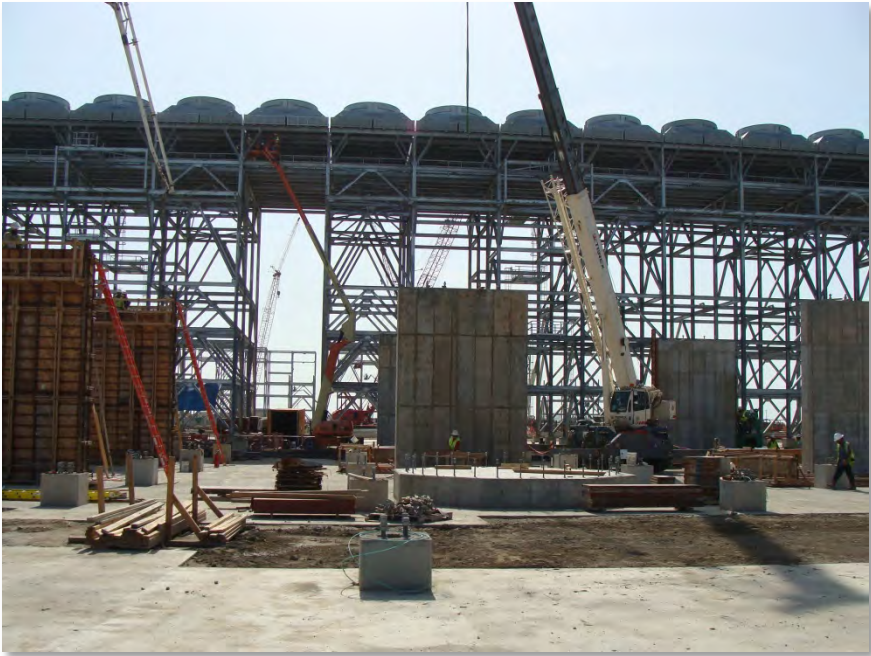
Train 1 area 131J (propane refrigeration) (29-July-2013)
