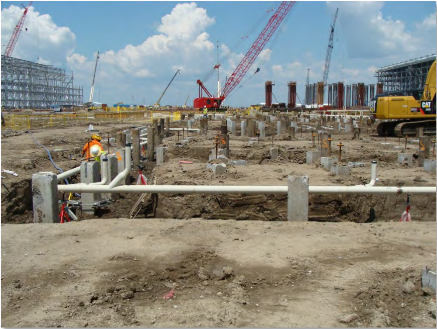
Train 2 132C (amine underground pipe) (23-Aug-2013)
