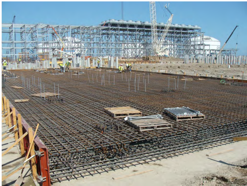
Train 2 area 132H (ethylene refrigeration cold box) (18-June-2013)
