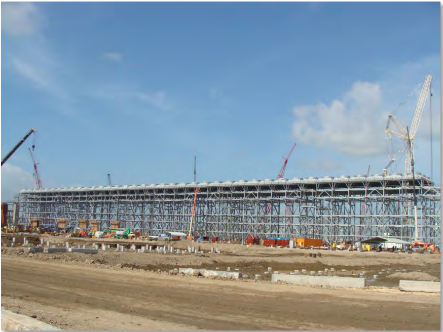
Train 1 area 131N (propane condenser) (23-July 2013)
