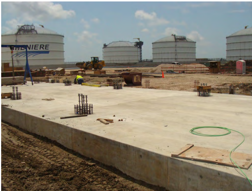
Train 1 area 131F (inlet facilities) (16-May-2013)
