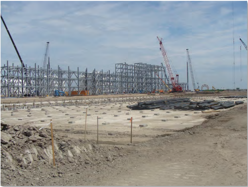
Train 1 Steel Area 132A (30-Apr-2013)
