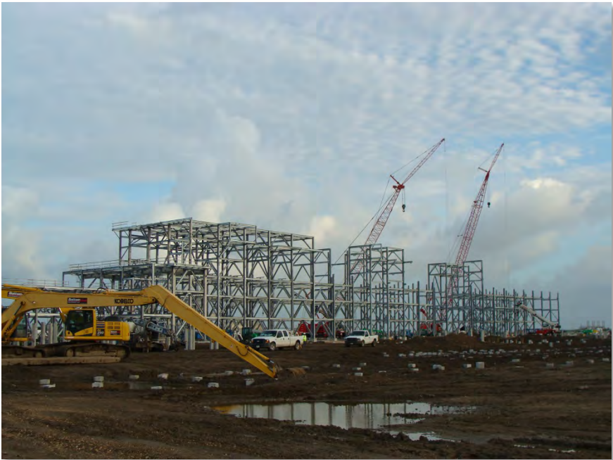
Train 2 area 132N (propane condenser) (22-July-2013)
