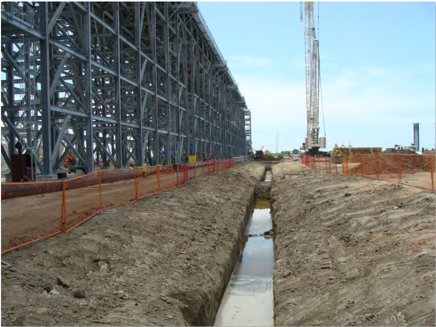
Train 1 131N01 (propane condensers underground pipe) (13-Aug-2013)
