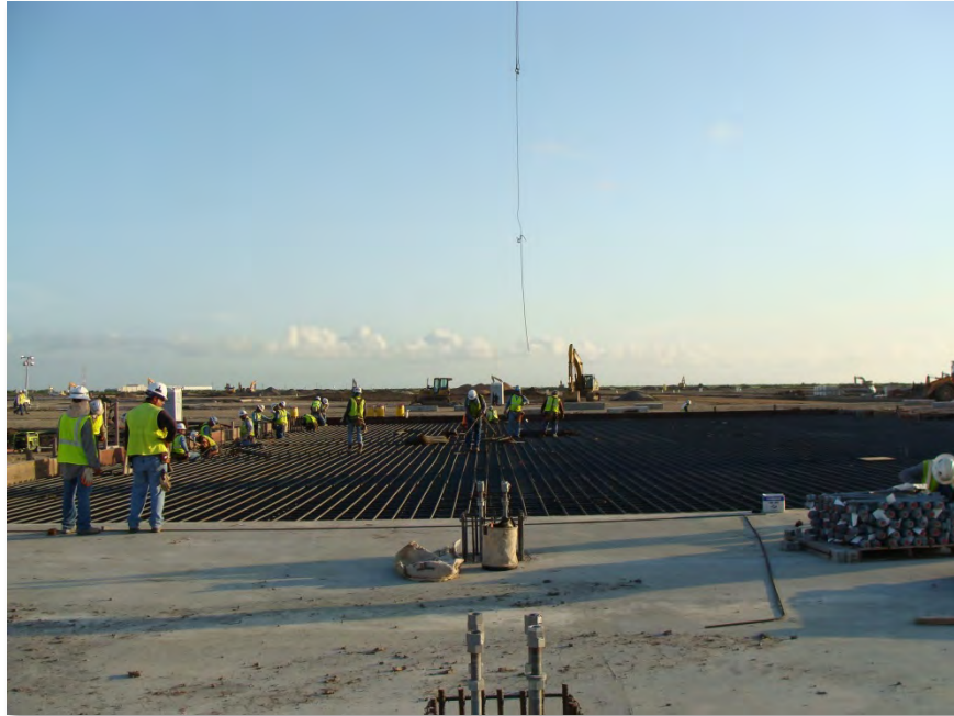
Train 1 area 131D (cryo rack) (06-June-2013)
