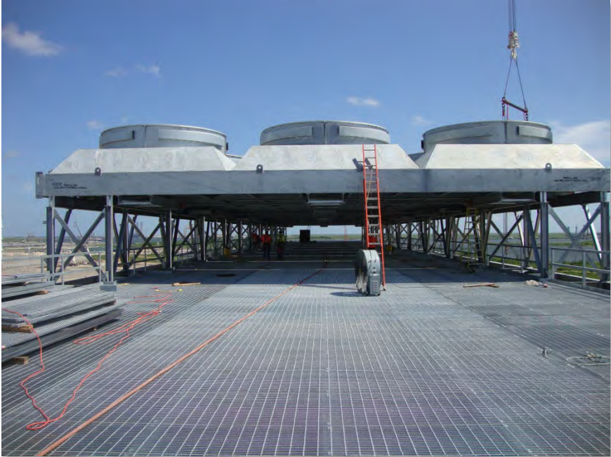
Train 1 area 131N (propane condenser) (17-June-2013)
