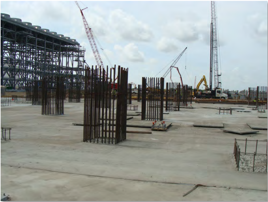
Train 2 area 132A01 (propane compressor) (26-July-2013)
