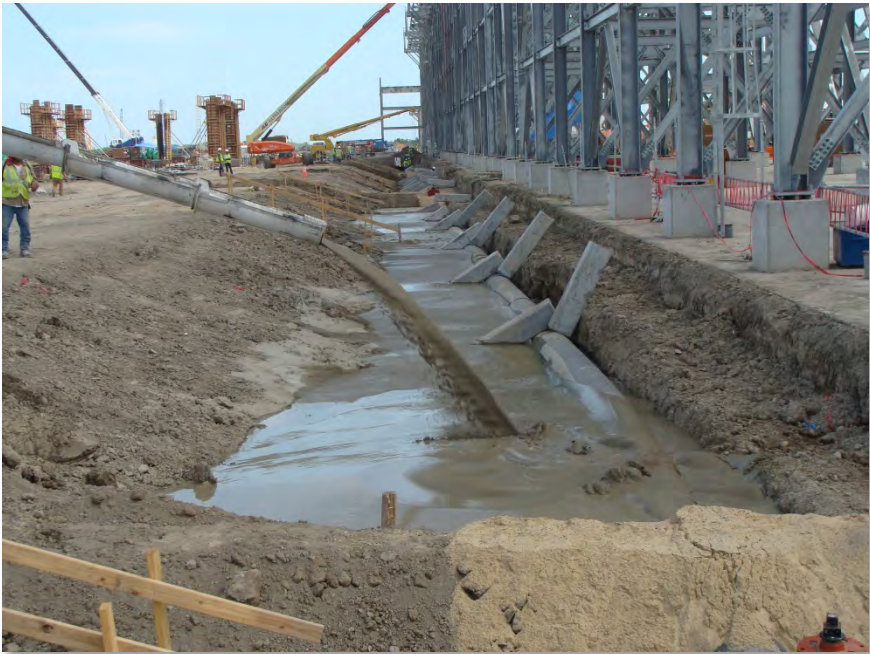
Train 1 area 131N (underground HDPE) (25-June-2013)
