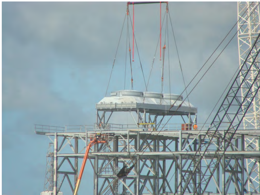
Train 1 area 131N (propane condenser) (10-June 2013)
