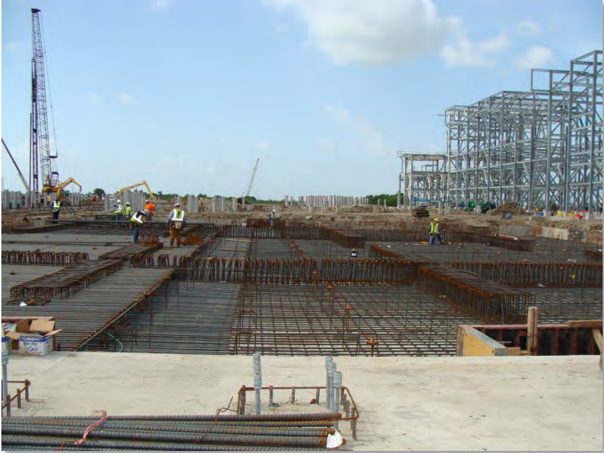
Train 2 area 132J (propane refrigeration) (23-July-2013)
