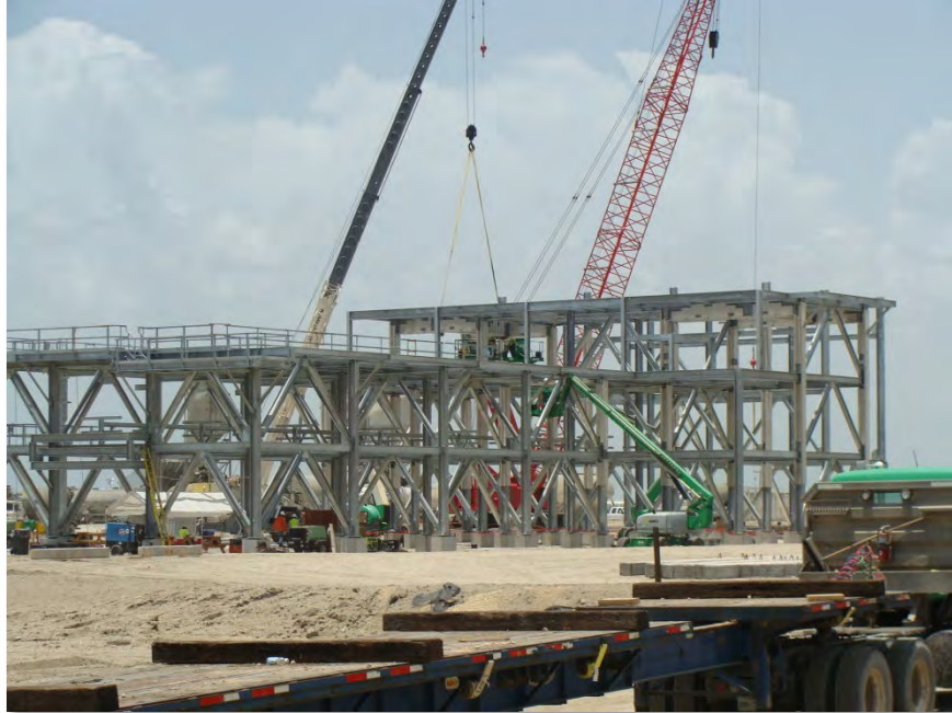
Train 2 area 132N (propane condenser) (20-June-2013)
