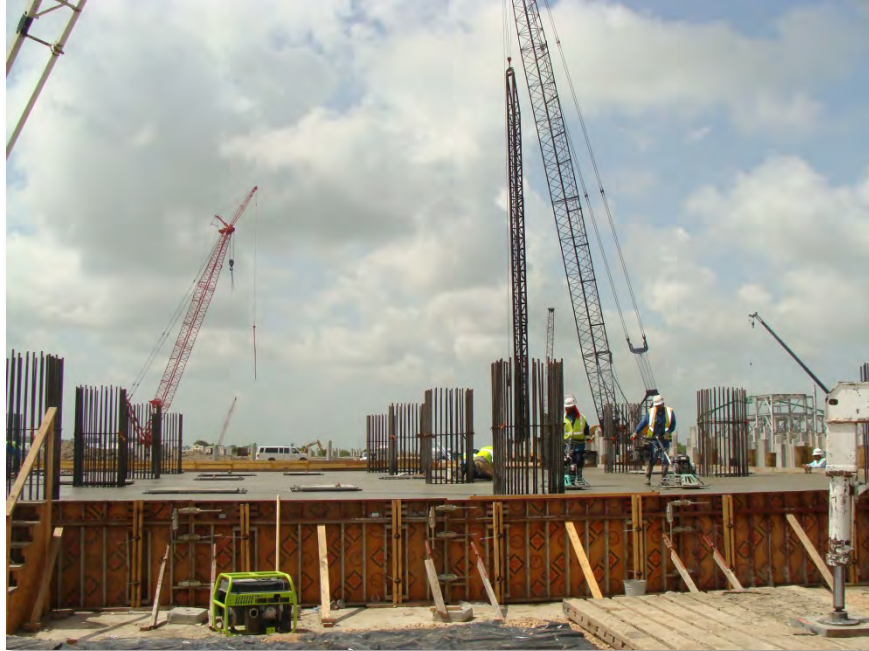
Train 2 area 132A01 (methane compressor) (11-June-2013)
