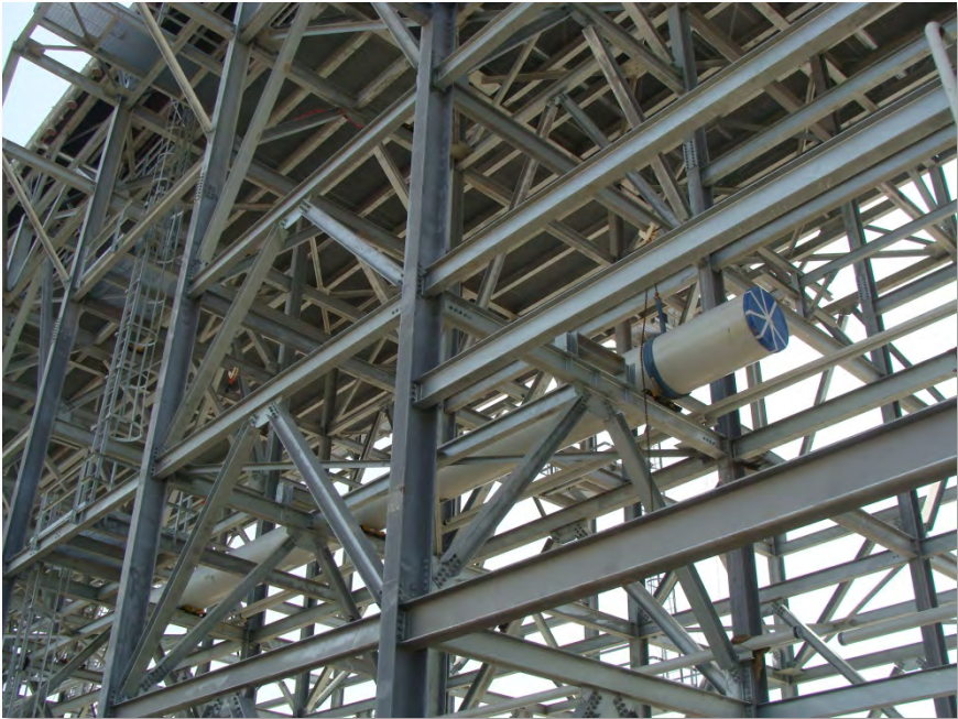
Train 1 131N01 (propane condensers aboveground pipe) (7-Aug-2013)
