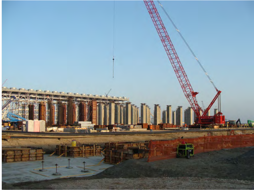
Train 1 131A01 (compressor columns) (19-Aug-2013)
