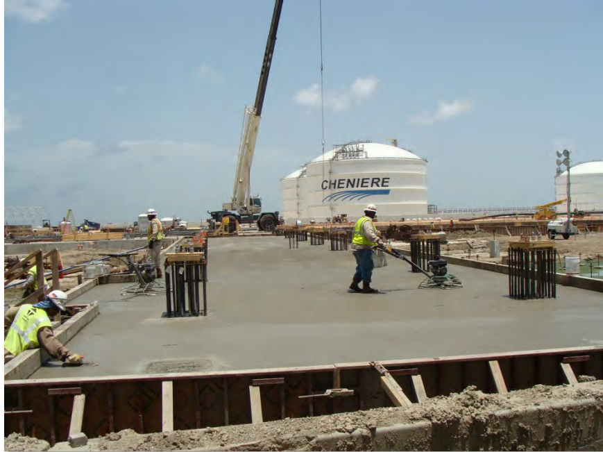
Train 1 area 131K (dehydration mercury removal) (20-June-2013)
