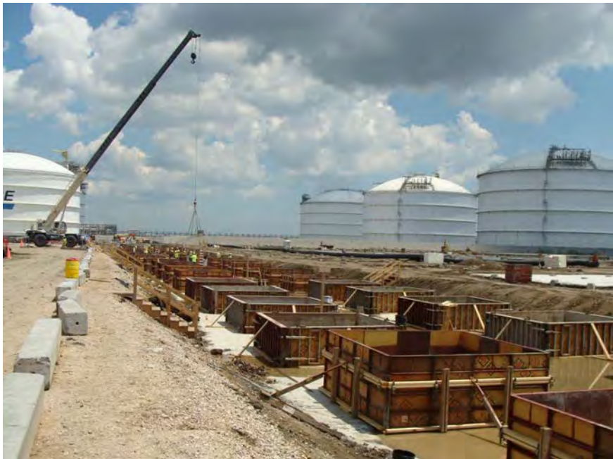
OSBL 135R07 (piperack utilities Train 1 & Train 2) (23-Aug-2013)
