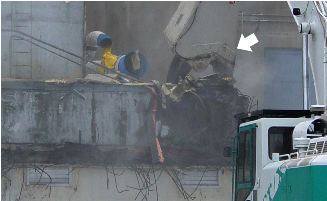
Exhibit 4-2: The Mechanical Shears Quickly Cut Up Reinforced Concrete Walls, Metal Sheet Walls, and Ventilation Ducting.
