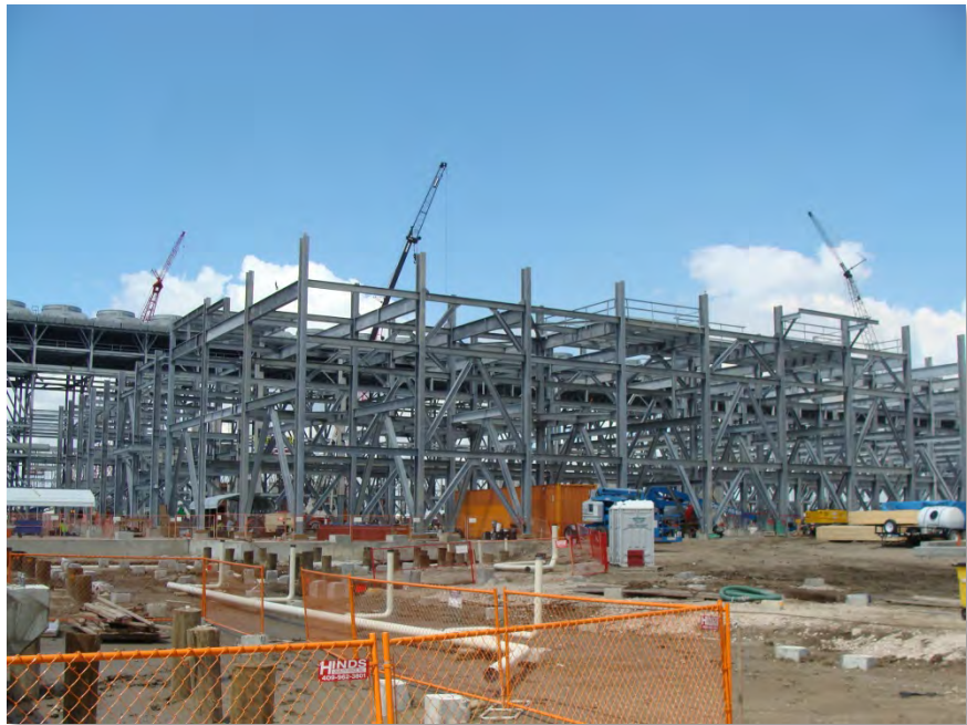
Train 1 131D01 (cryo air coolers piperack) (24-Sep-2013)
