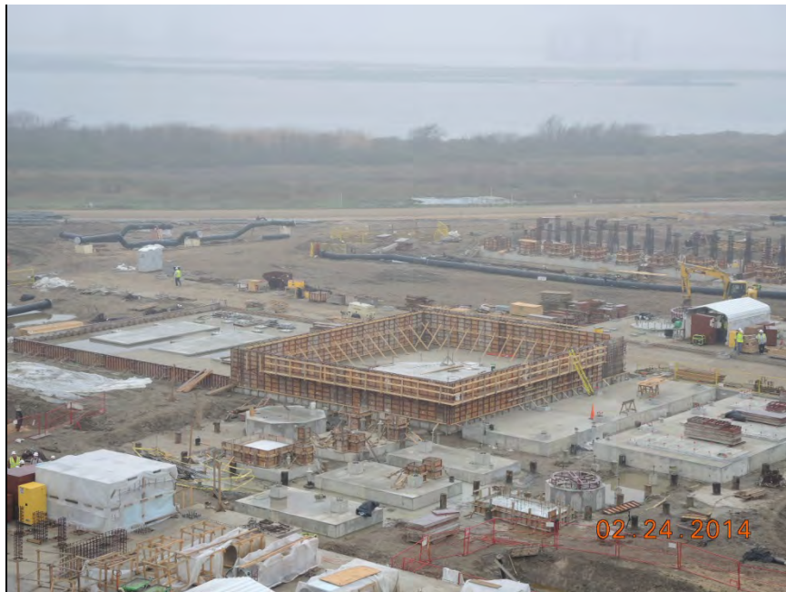
Train 2 132B01 (amine storage area and thermal oxidizer) (24-Feb-2014)
