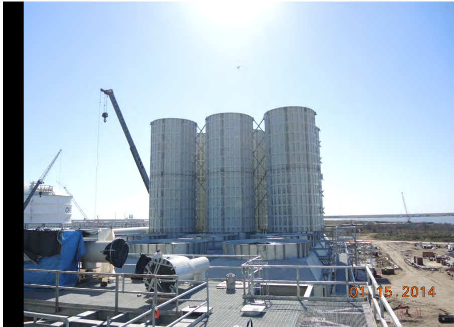
Train 1 131N01 (propane condenser subcooler stack) (15-Jan-2014)
