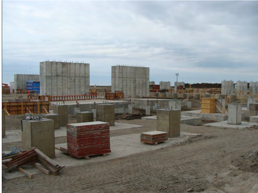
OSBL Refrigerant Storage 18-Nov-2013
