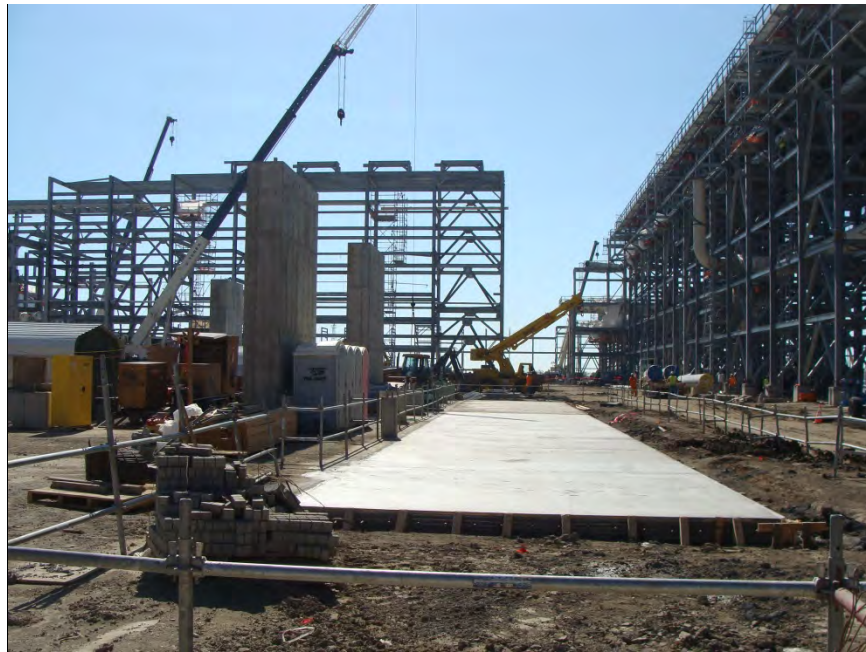
Train 2 (propane refrigeration) (15-Nov-2013)
