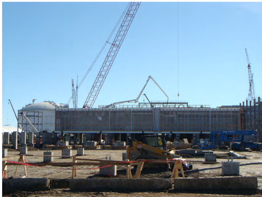
Train 1 (compressor substation)
