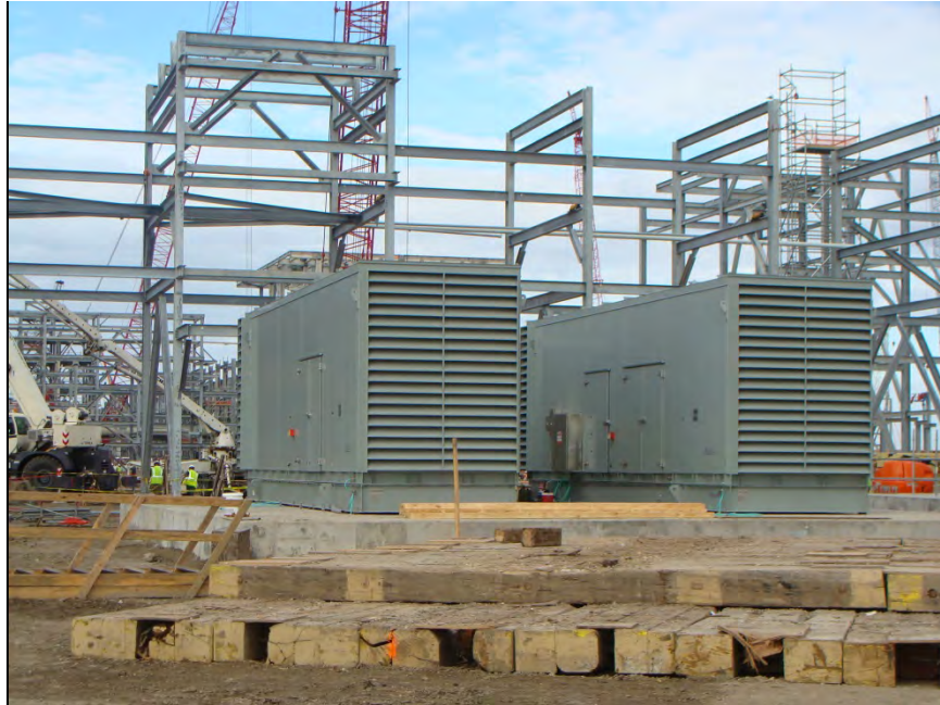
OSBL (utility substation emergency generator)
