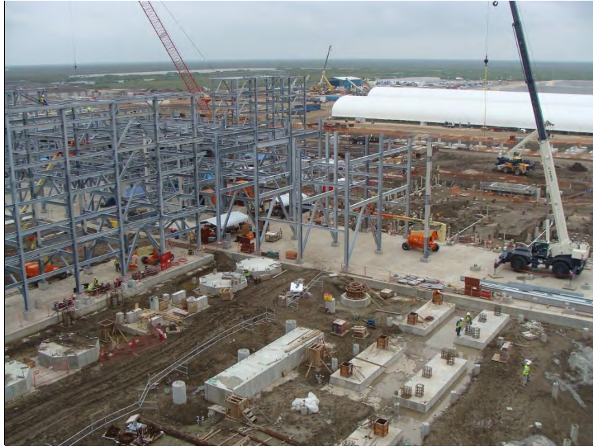
Train 1 (dehydration mercury removal) (22-Oct-2013)
