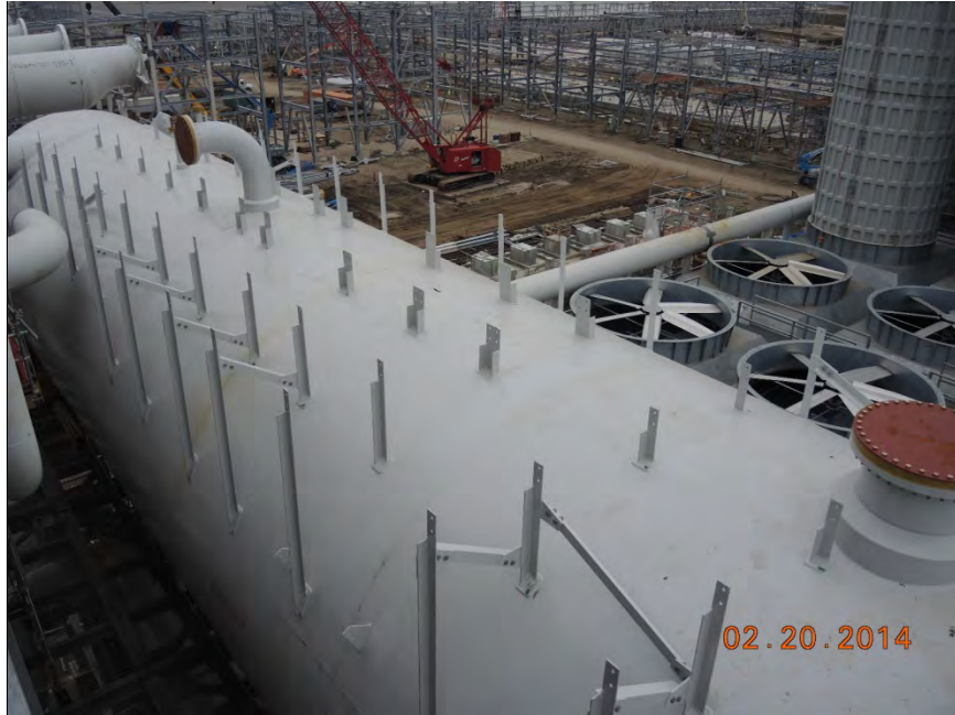
Train 1 131N01 (propane rack accumulator set) (20-Feb-2014)
