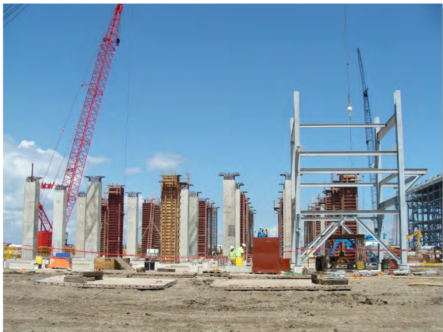
Train 2 132F01 (inlet gas and fuel gas) (24-Sep-2013)
