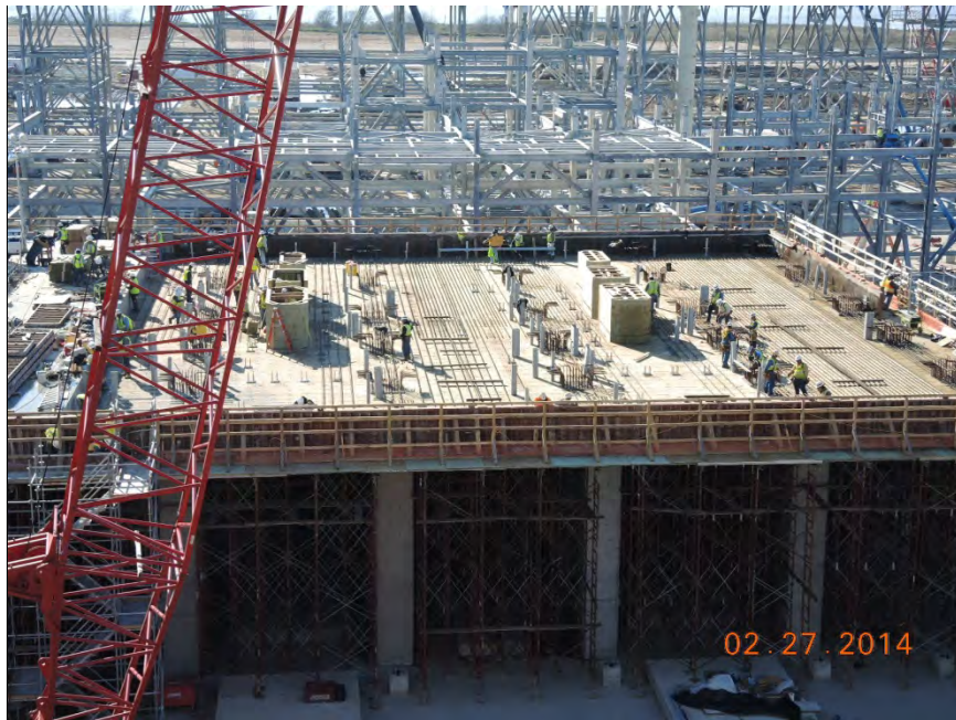
Train 2 132A01 (compressor methane tabletop) (27-Feb-2014)
