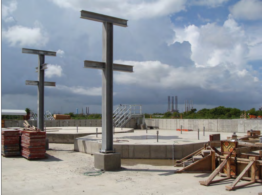
OSBL 135C01 (utilities waste water and solvent storage) (23-Sep-2013)
