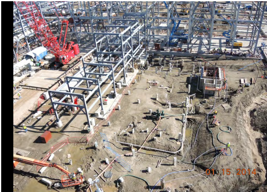
Train 1 131L01 (hot oil surge drum and sump) (15-Jan-2014)
