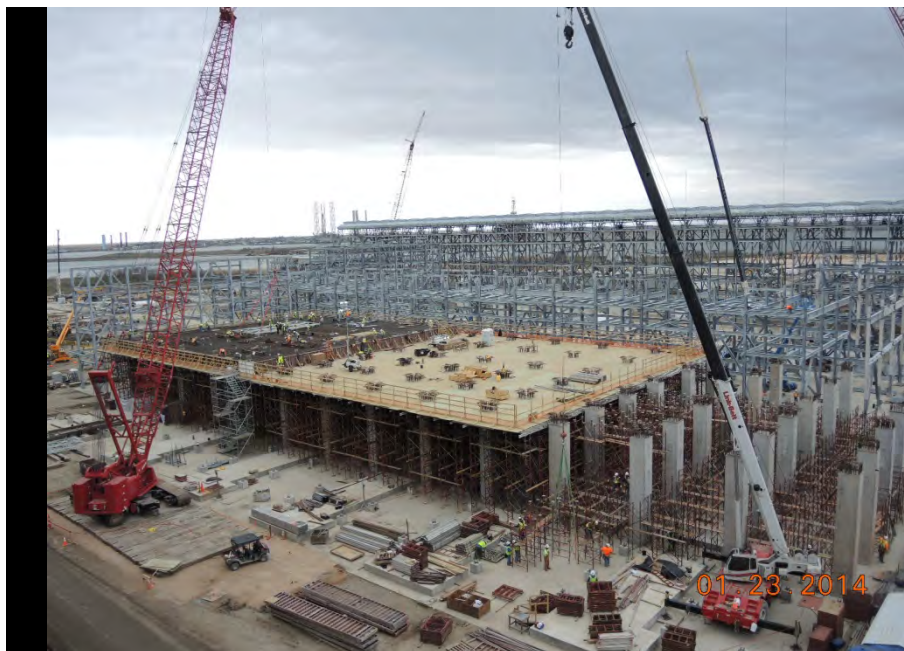
Train 2 132A01 (compressor propane and ethylene tabletops) (23-Jan-2014)
