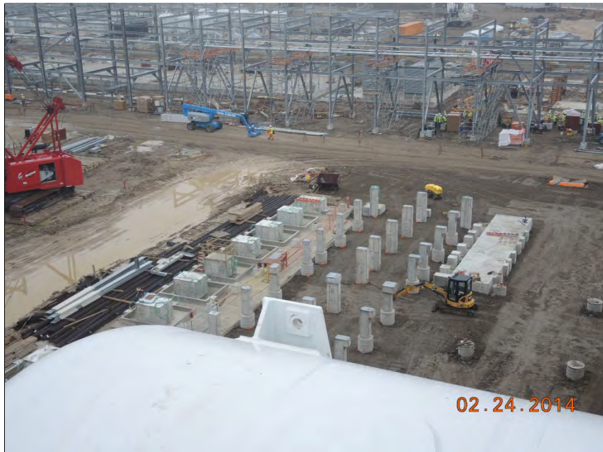
Train 1 131N02 (propane substation) (24-Feb-2014)
