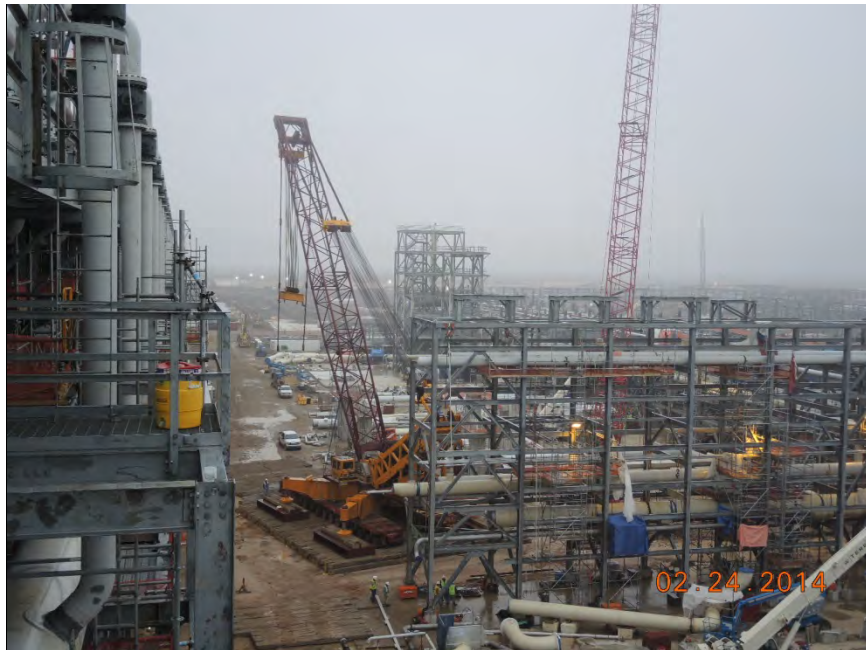
Train 1 131K01 (dehydration mercury removal) (24-Feb-2014)
