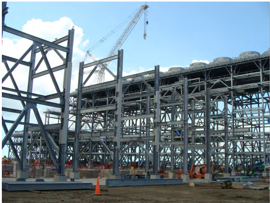
Train 1 131K (dehydration mercury removal) (24-Sep-2013)
