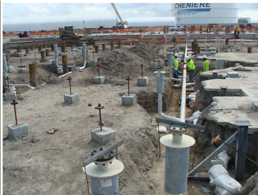
Train 1 131C01 (amine underground pipe) (18-Sep-2013)
