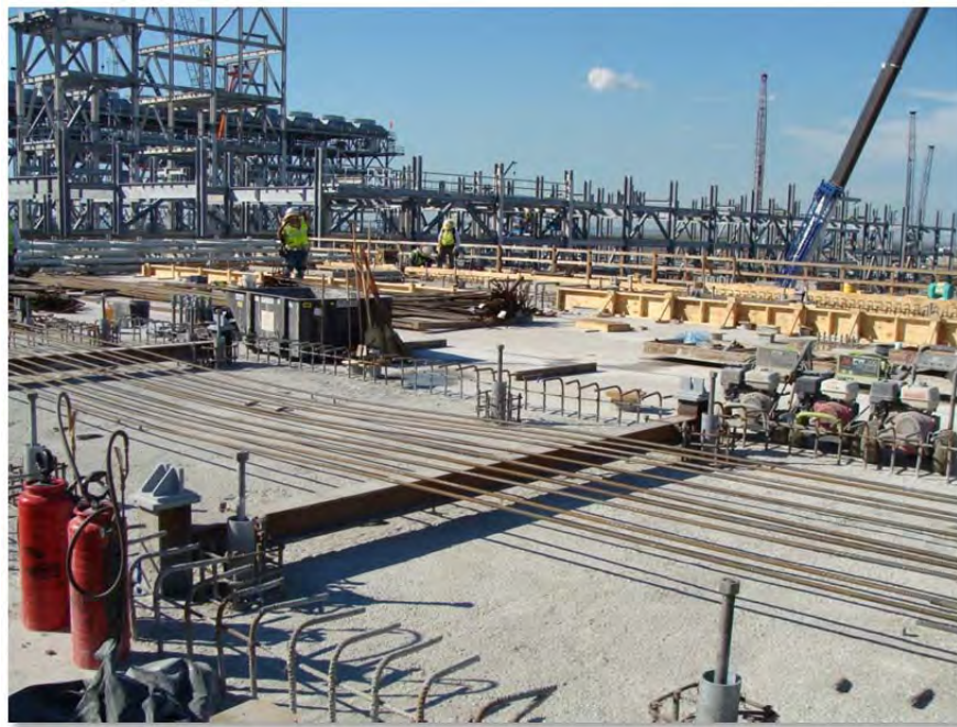
Train 1 (compressor area ethylene tabletop) (24-Oct-2013)
