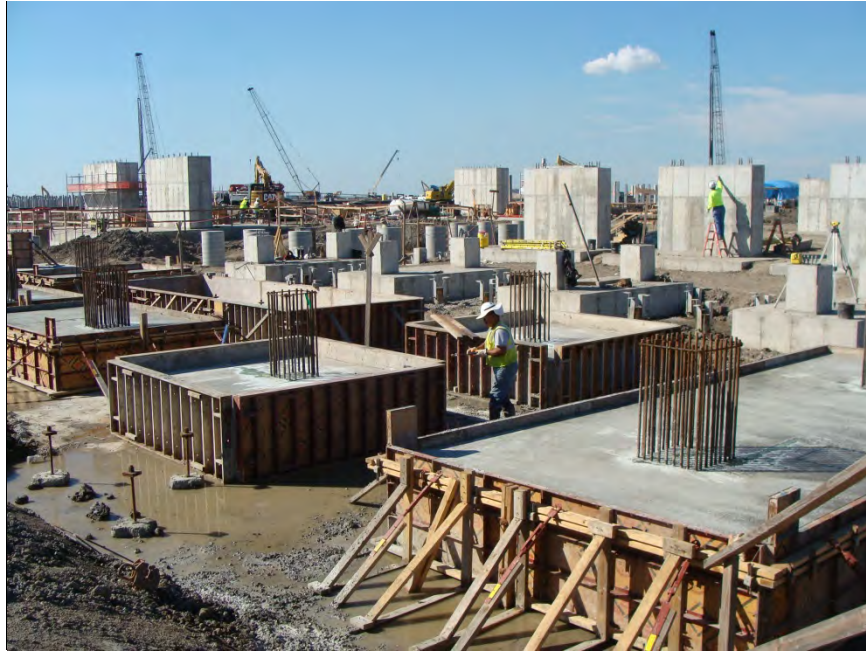
OSBL (refrigerant storage) (24-Oct-2013)
