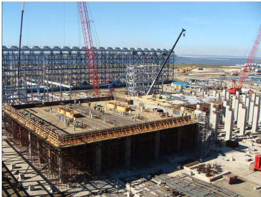
Train 2 (compressor propane tabletop)
