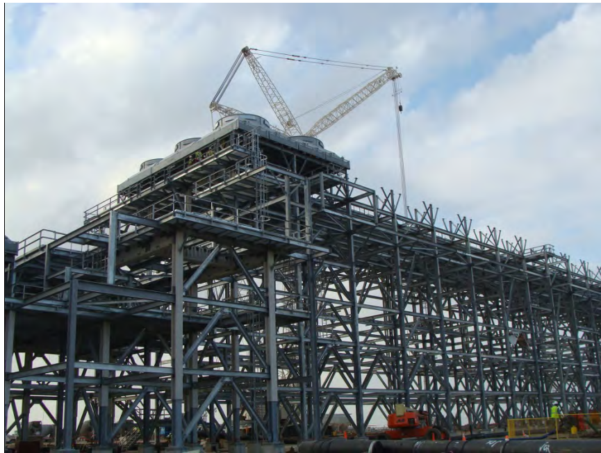
Train 2 (propane condensers) (5-Nov-2013)
