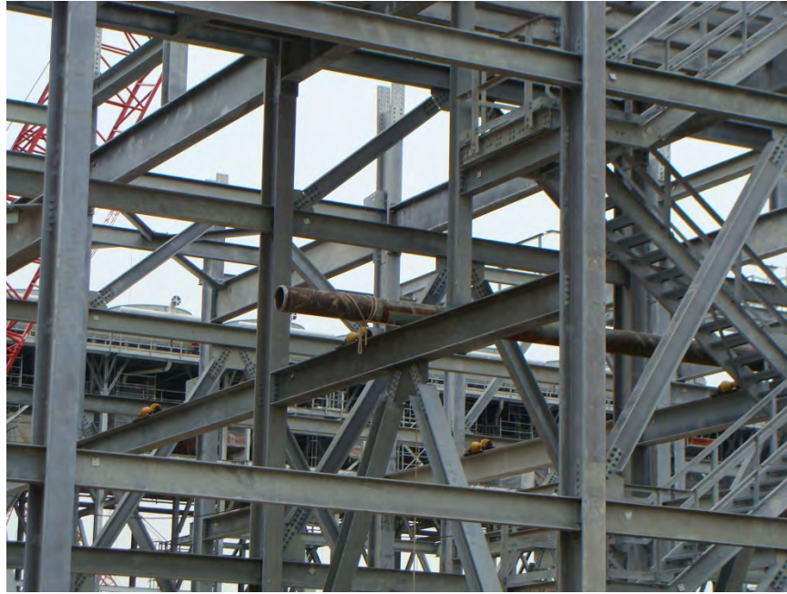
Train 1 (cryo air coolers piperack AG pipe)
