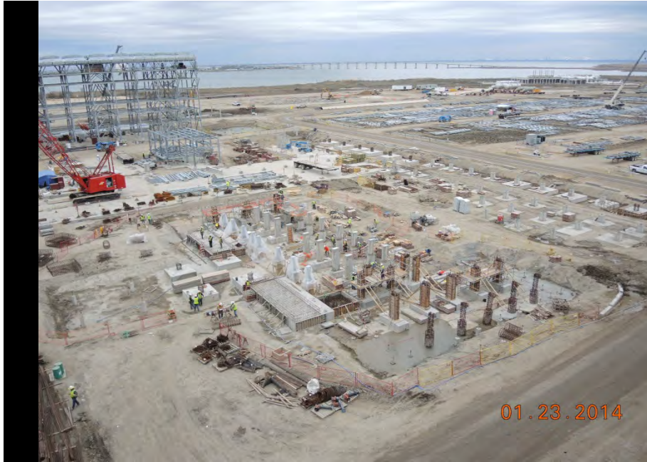
Train 2 132A02 (compressor substation) (23-Jan-2014)
