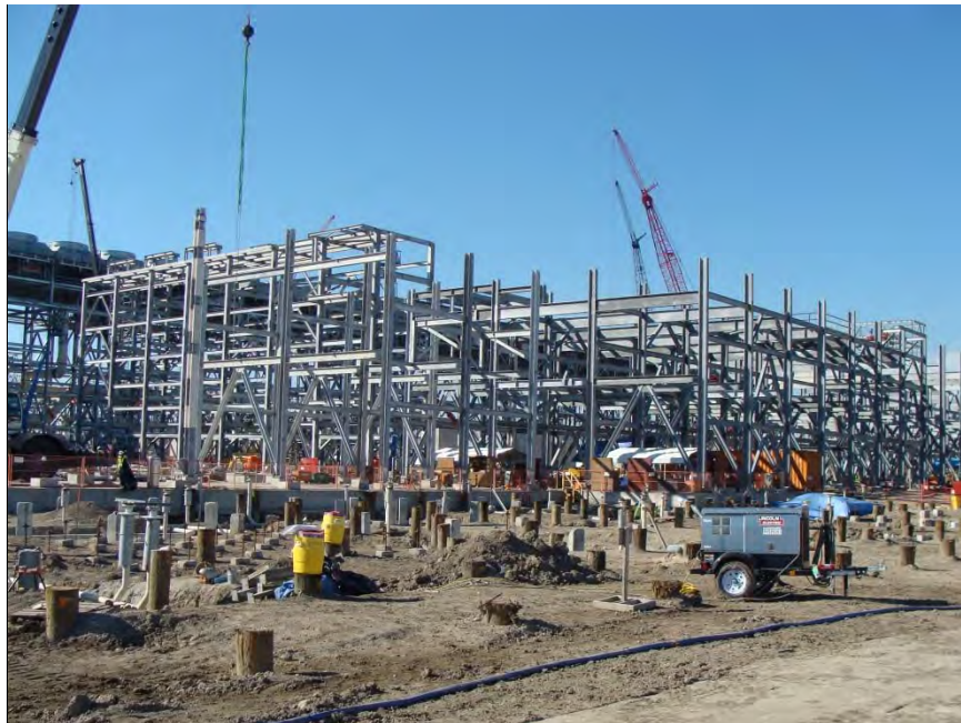
Train 1 (cryo-rack piperack) (24-Oct-2013)
