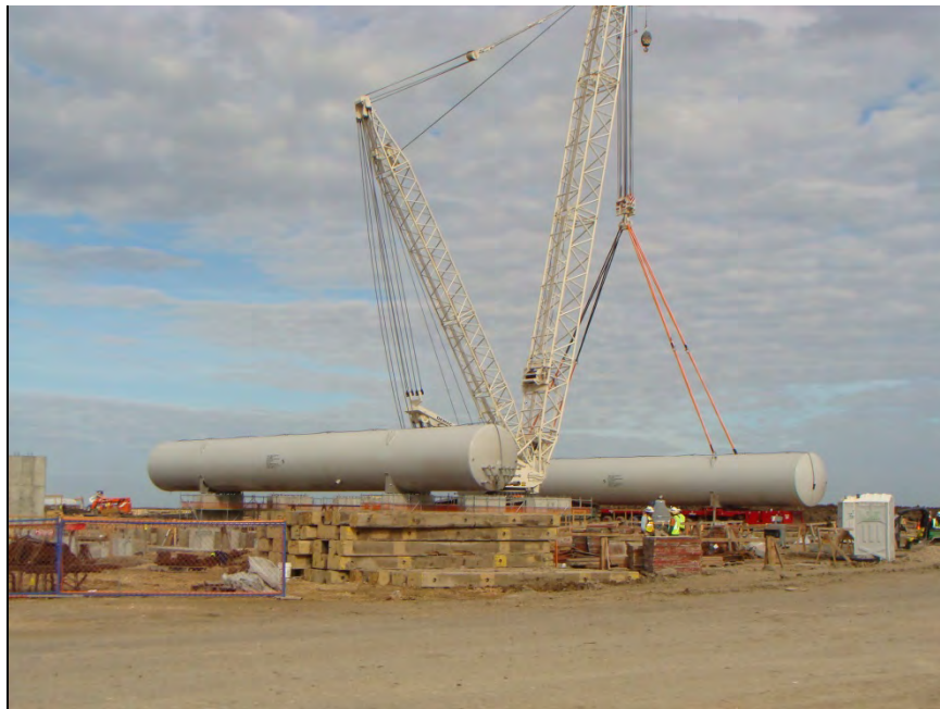
OSBL (refrigerant storage)
