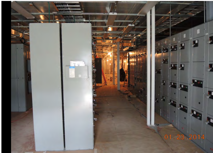
Train 1 131A02 (compressor substation inside) (23-Jan-2014)
