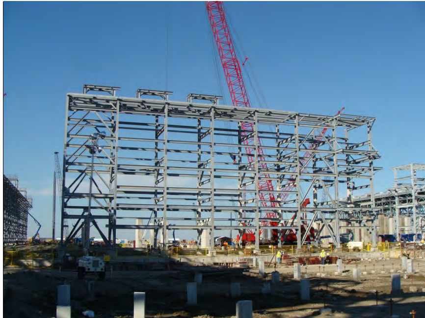
Train 2 (dehydration mercury removal) (24-Oct-2013)
