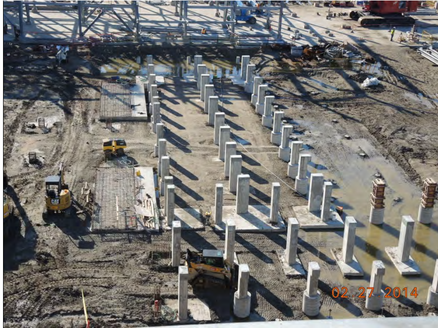
Train 2 132A02 (compressor substation) (27-Feb-2014)
