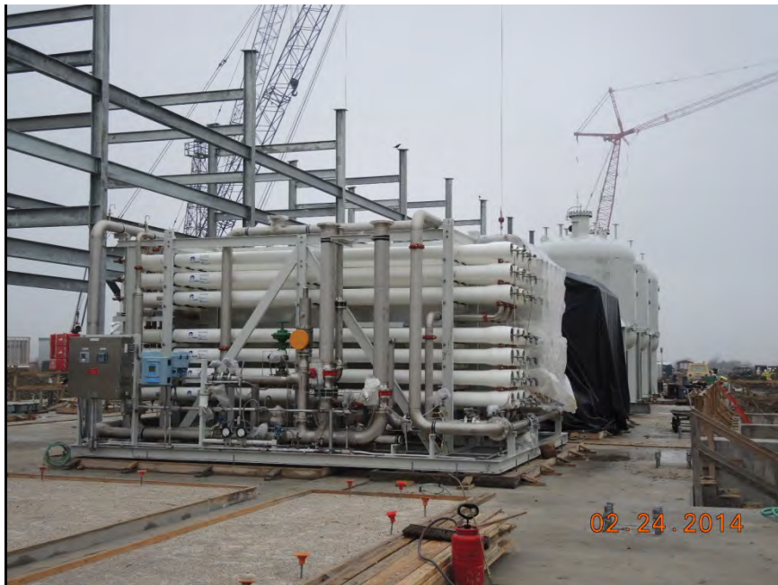
OSBL 135F01 (water treatment area) (24-Feb-2014)
