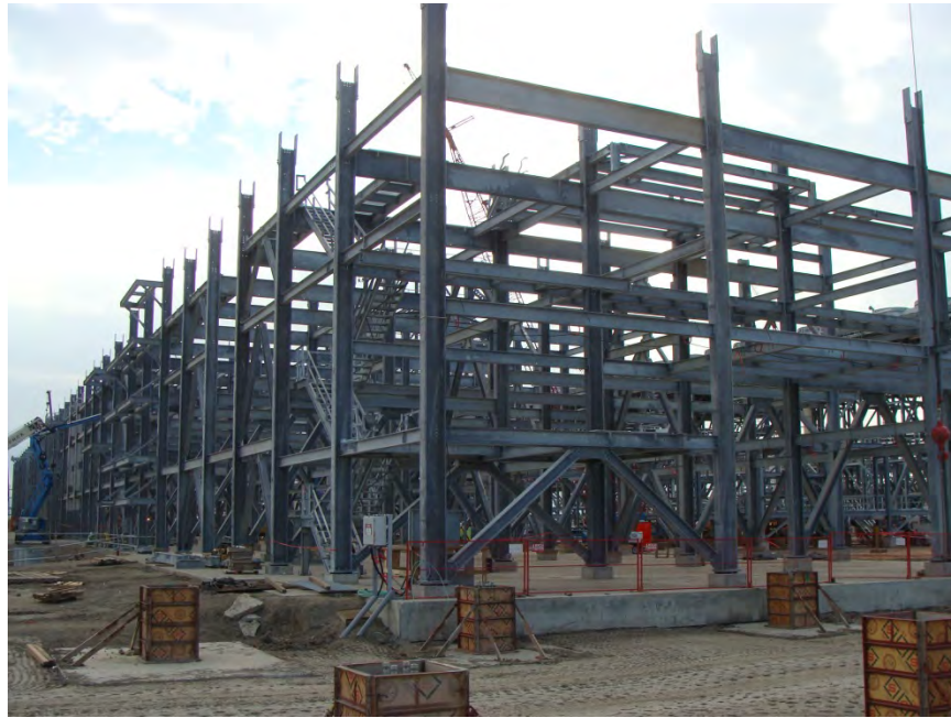
Train 1 (cryo air coolers piperack) (18-Nov-2013)
