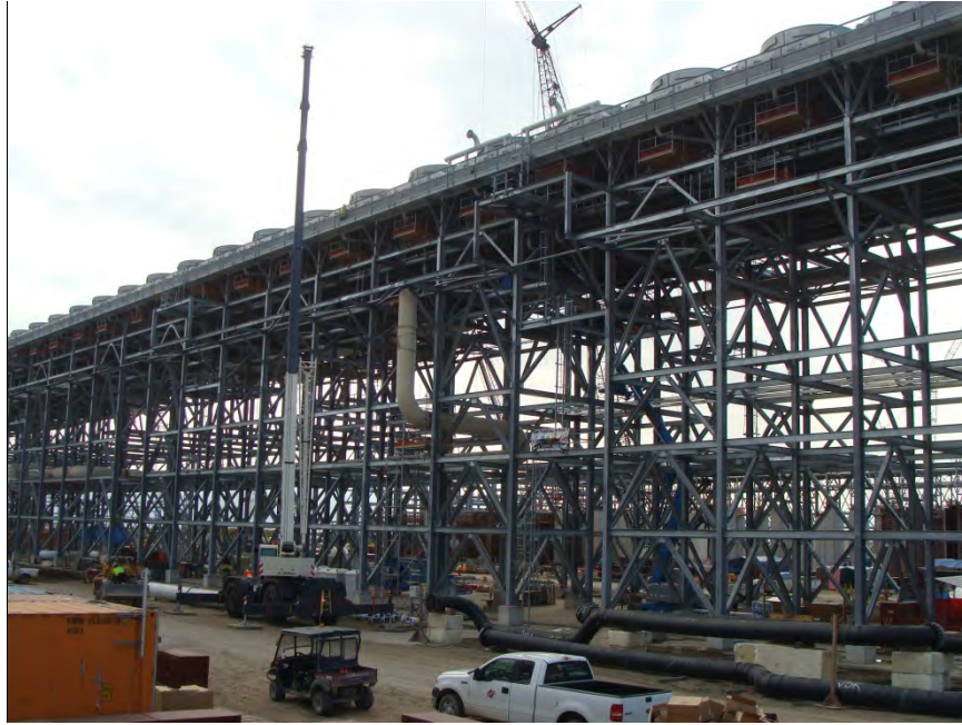
Train 1 (propane condenser) (18-Nov-2013)
