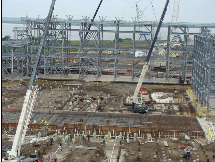
Train 2 (AGRU coolers/pipe rack) (22-Oct-2013)
