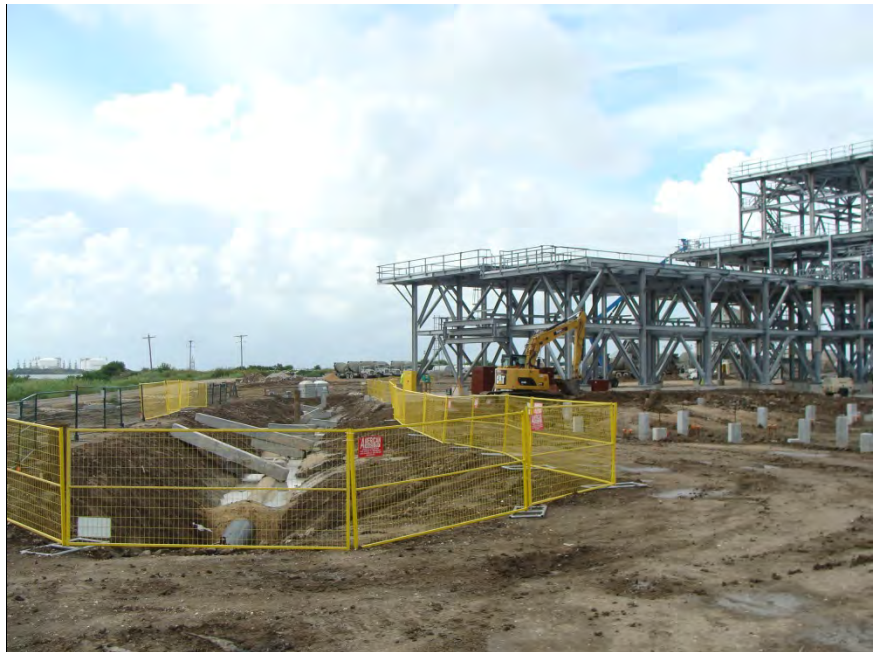
Train 2 132U (FW underground pipe) (19-Sep-2013)
