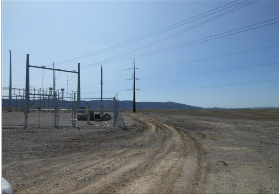
Figure 2-2. Area of the Proposed Hooper Springs Substation (Threemile Knoll Substation is to the left)
