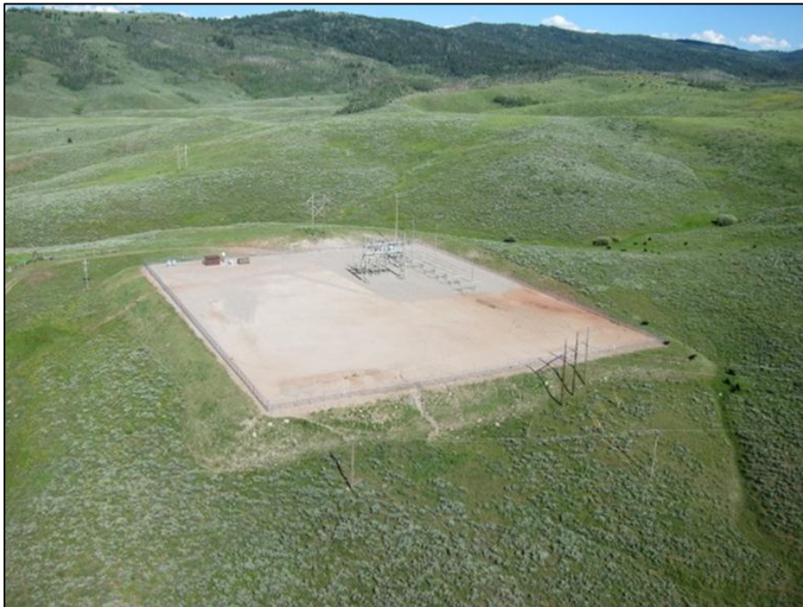
Figure 2-3. Existing Lanes Creek Substation
