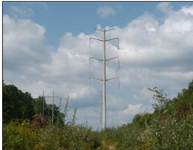
Figure 3-17. Typical Double-Circuit Steel Pole Transmission Line
