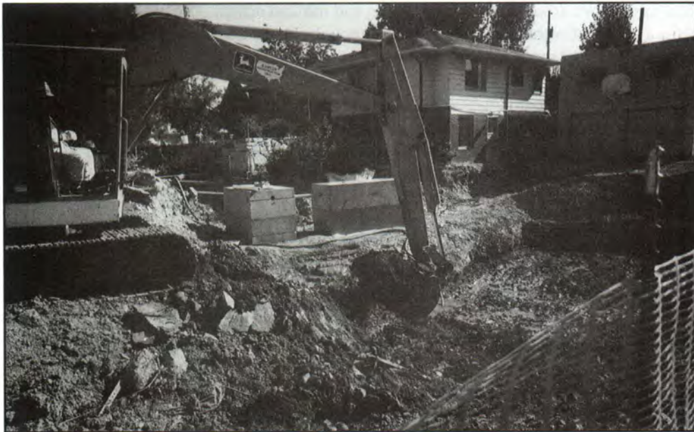
Excavation of uranium mill tailings from a residential septic system, Grand Junction, Colorado, 1993. Uranium mining produced large volumes of a sandlike byproduct called "mill tailings," containing both toxic heavy metals and radioactive radium and thorium. Uranium-mill tailings account for a small fraction of the radioactivity in the byproducts of weapons production, but they constitute 96 percent of the total volume of radioactive byproducts for which the Environmental Management program is responsible. Because uranium mills typically piled tailings without covers or containment, some material was spread by wind or water. Life-cycle planning is an effective way to understand and predict the importance of such precautions and, ultimately, is an effective method for ensuring long-term cost savings.
