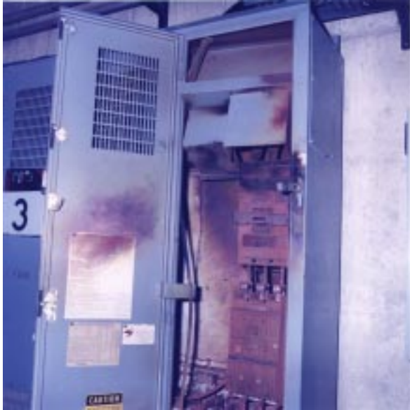
The Damaged Bus Bar Cover
