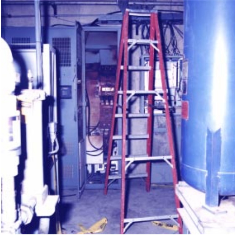
Exhibit 2-1. View of Accident Location
