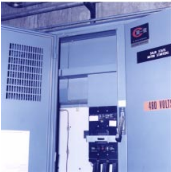
Similar Intact Bus Bar Cover
