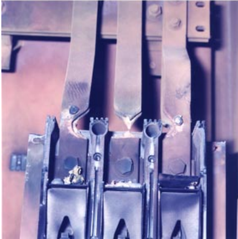
Exhibit 2-2. View of Bus Bar after Electrical Blast
