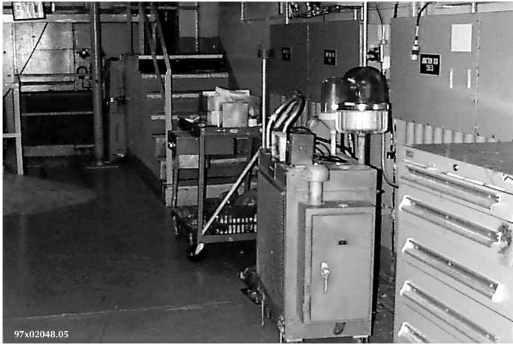
Exhibit 2-5 Warm Gang Valve Corridor Continuous Air Monitor
