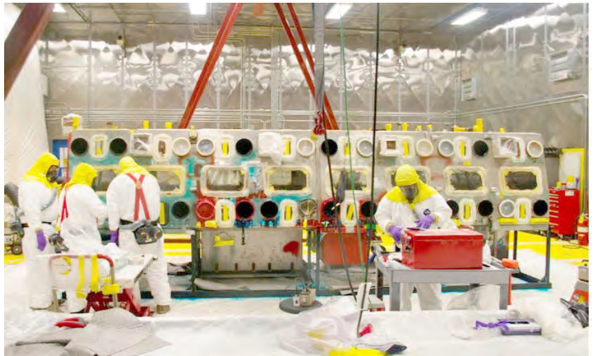
Advanced techniques allowed crews at Los Alamos National Laboratory to decontaminate large boxes of waste so they could be shipped as mixed low-level, rather than transuranic, waste.
