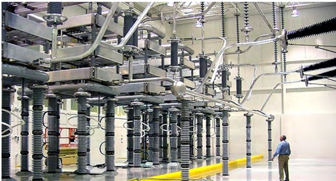
Bonneville Power Administration completes the modernization of the Celilo Converter Station (Dalles, Oregon) located at the northern end of the 846 mile direct Pacific Intertie that connects the Pacific Northwest with Los Angeles, California. The modernization project uses solid-state silicon chips that will allow the system to work cooler, safer and be ecologically improved.
