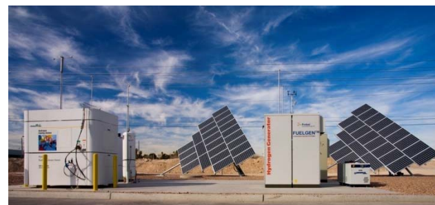
The Las Vegas Nevada renewable hydrogen generation/distribution system is composed utilizing 13 kg/day PEM electrolyzers http://www.protononsite.com/technology/hydrogen-fueling-systems.html
