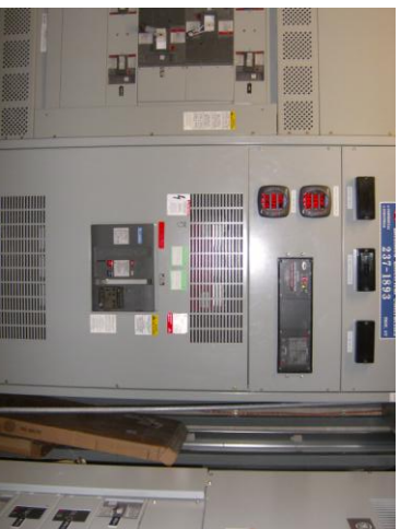
Generator – CHP system at One Penn Plaza
