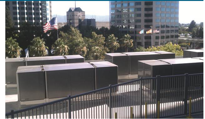
1.2 MW Bloom Fuel Cell Installation at Adobe Headquarters in San Jose, California Adobe expects to reduce its carbon footprint by approximately 121.5 million pounds over the next 10 years
