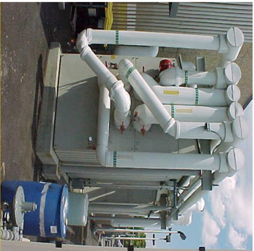
During the cooling season, the high-grade waste heat from the fuel cells is used by two lithium bromide absorption chillers, contributing about 33% of the energy required for cooling.
