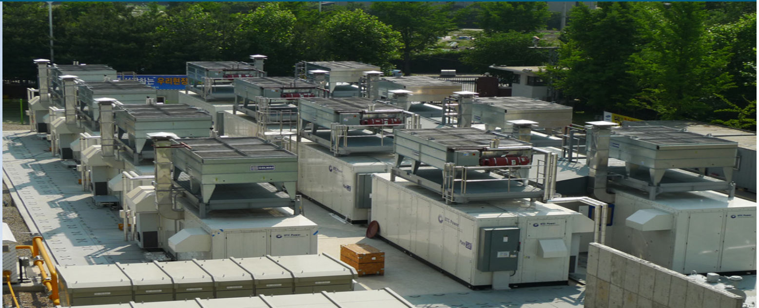
Twelve UTC Power 400 kW fuel cell systems purchased by Samsung Everland. The fuel cells are installed at a GS Power plant in the Town of Anyang, just outside Seoul. GS Power uses the electricity from the fuel cells to provide power for about 5 percent of Anyang's population. Photo courtesy of UTC Power
