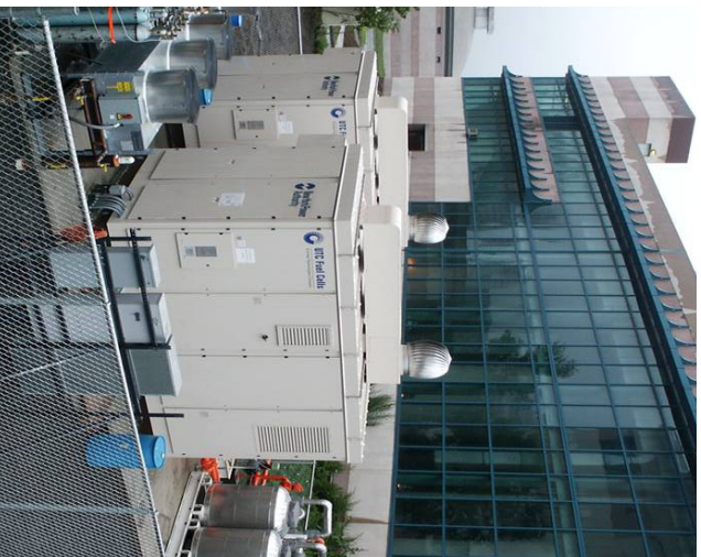
Fuel cells in a combined heat and power installation, using biogas.
