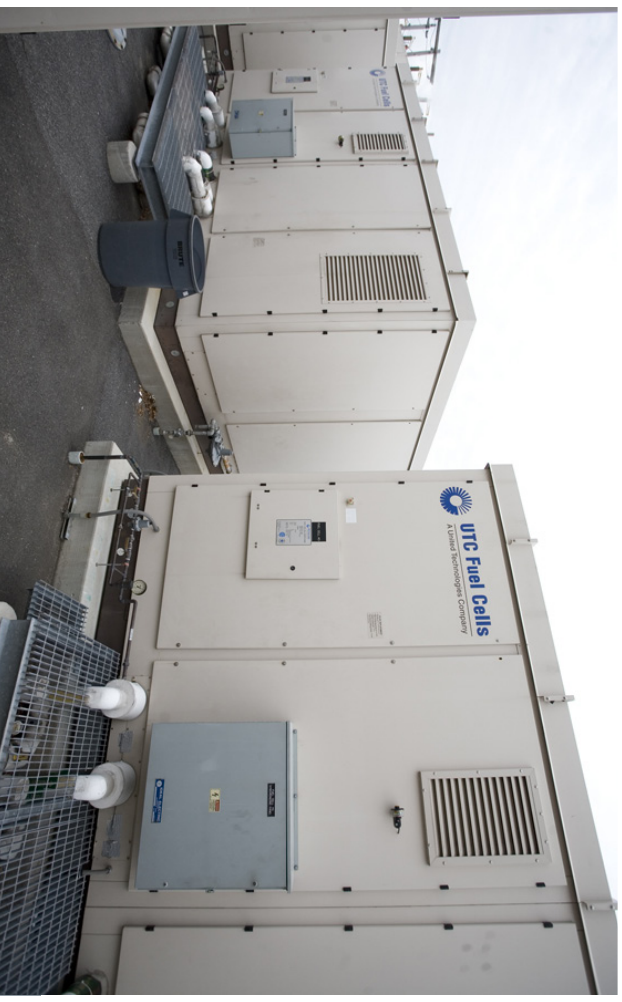
A fuel cell CHP system provides primary power, heating, and cooling for Verizon's Central Office.
