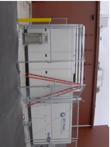
400 ton power plant on the 12th floor roof overcropping
