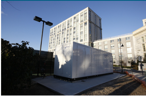
A UTC Power PAFC 400 kW fuel cell installed at the Octagon building on Roosevelt Island in New York. The Octagon is a Leadership in Energy and Environmental Design®(LEED) Silver 500-unit apartment community that made green history by becoming the first residential building in the State of New York to be powered and heated by a 400 kW fuel cell from UTC Power.
