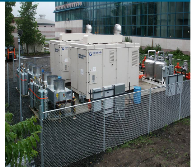
UTC Fuel Cells PAFC installation at NYSERDA
