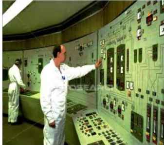
Plant Status Display
