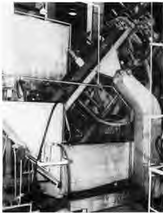
ALPHA 1 UNIT IN WASHSTAND / Part of the process of recovering the uranium-tetrachloride charge that did not reach the receiver.
