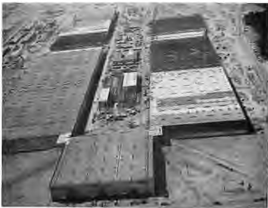
K-25, THE GASEOUS-DIFFUSION PLANT, UNDER CONSTRUCTION / The U-shaped building contained thousands of pumps and converters for concentrating uranium 235. Service facilities are in the center.
