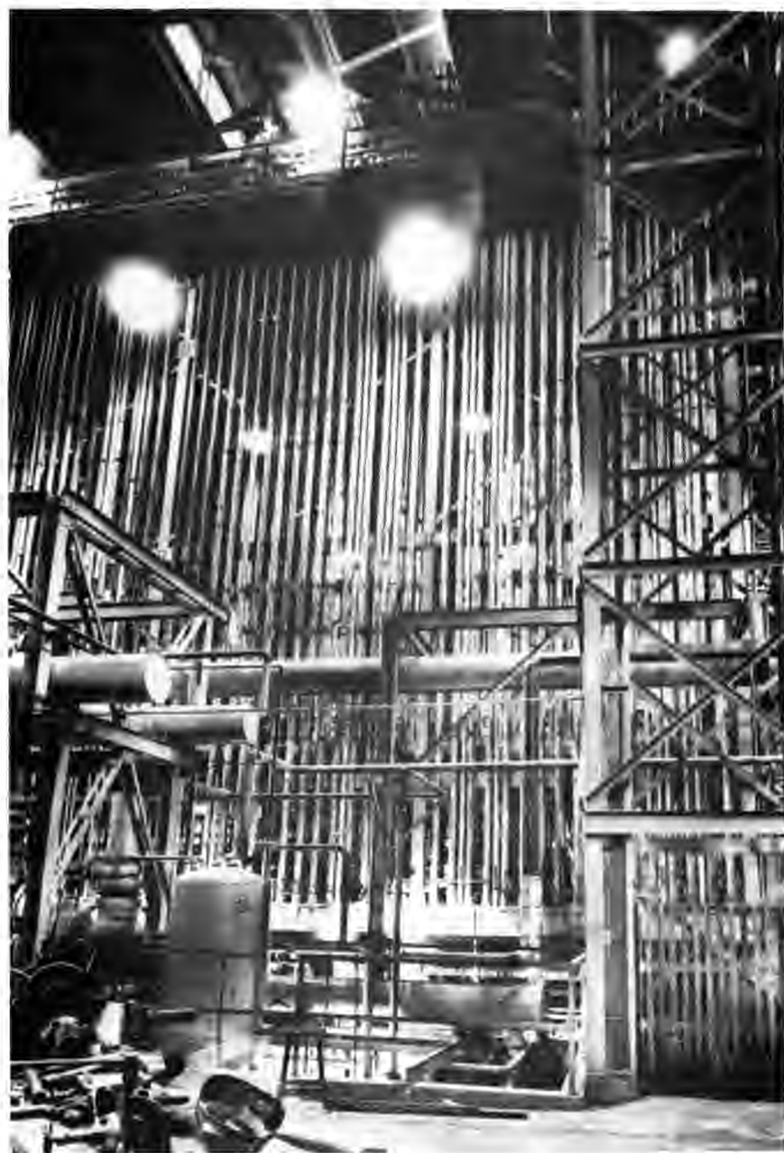
INTERIOR OF S-50, LIQUID-THERMAL-DIFFUSION PLANT / A few of the 2,142 identical 48-foot process columns that were housed in a building 522 feet long, 82 feet wide, and 75 feet high.
