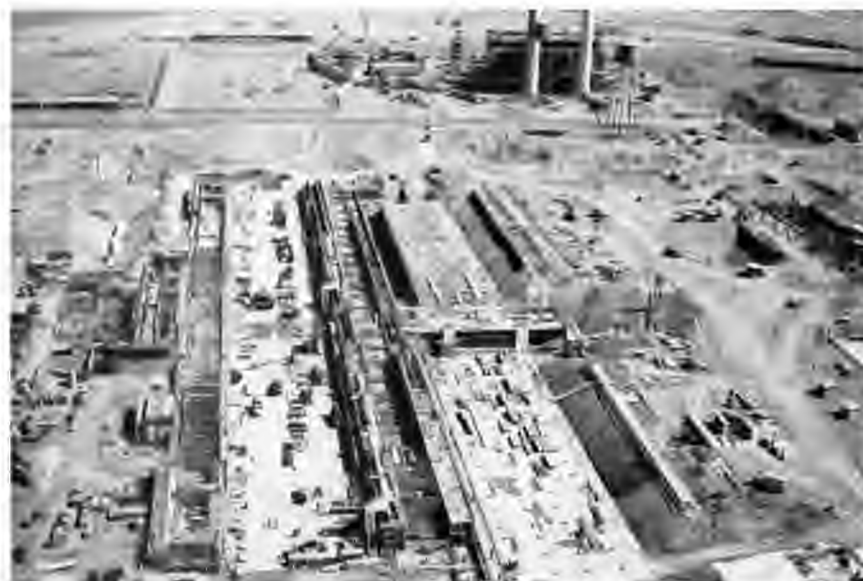
FILTER PLANT FOR THE HANFORD D PILE, JUNE 20, 1944 / The water-treatment system for each of the three production piles was comparable to a large municipal plant. The power plant is in the background and the pile building out of view to the right.
