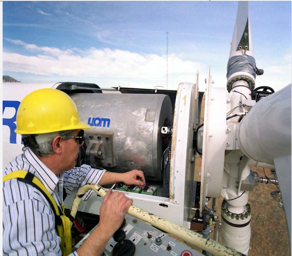
Photo by Warren Gretz, NREL 04119
