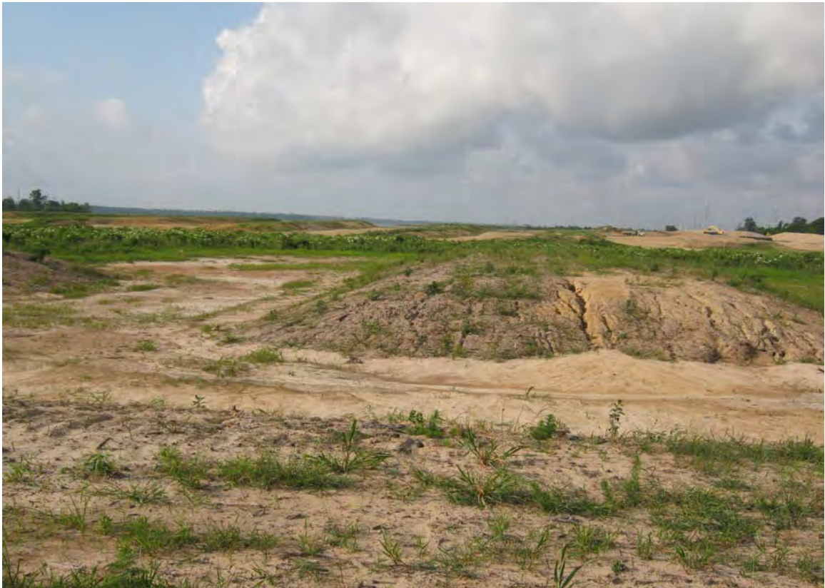
Figure 20. South view of mechanical impact at southern origin point of pipeline.
