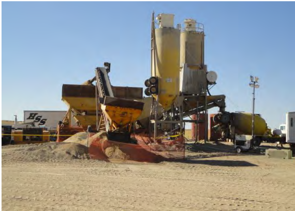
Figure 2-2 Typical Temporary Concrete Batch Plant
