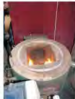
Small wood chip boiler heating a greenhouse
