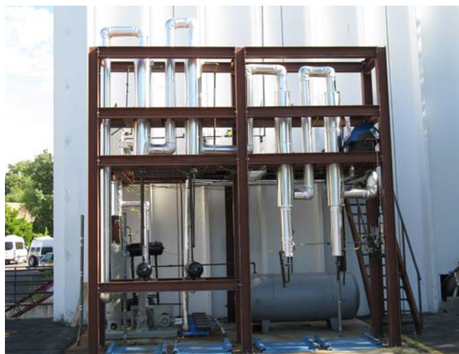
Separations Unit and Support Stand of the C-SOS Pilot Plant
