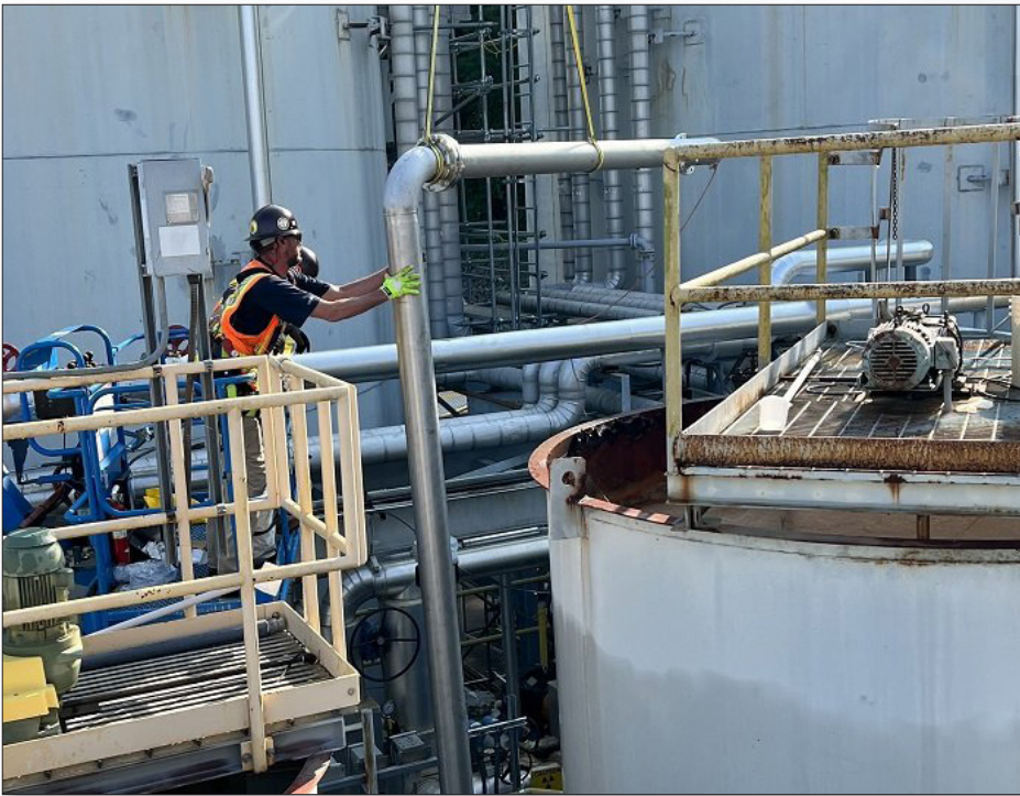
Oak Ridge crews installed approximately 5,500 feet of new piping as part of a project at the Liquid and Gaseous Waste Operations system. The work required 5,000 hours of welding to complete the nearly two miles of welded lines.
