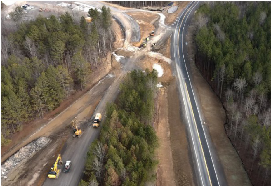
Early site preparation activities for Oak Ridge's Environmental Management Disposal Facility were completed this spring. One of the major tasks involved moving Bear Creek Road and Haul Road.
