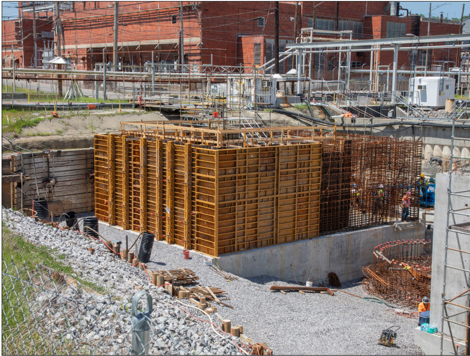
Work is currently underway at the Mercury Treatment Facility (MTF) at Y-12. MTF is one of the projects for which ORSSAB members listed support in its recommendations to DOE on OREM's FY 2026 budget priorities.
